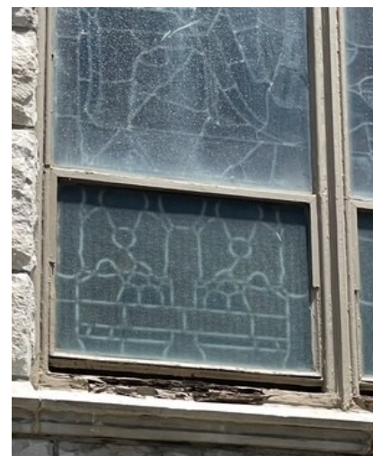
Wood rot visible under window
