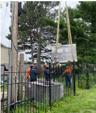
New air conditioner installed
