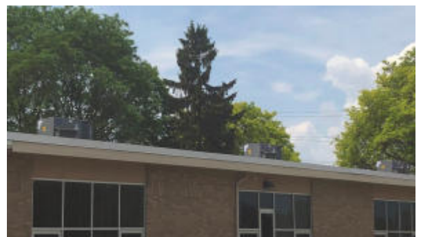
New units installed
