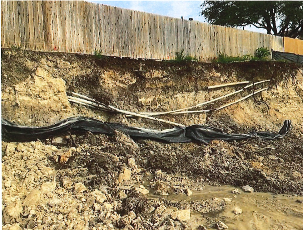
Damage at construction site – 300 Venture Blvd North
