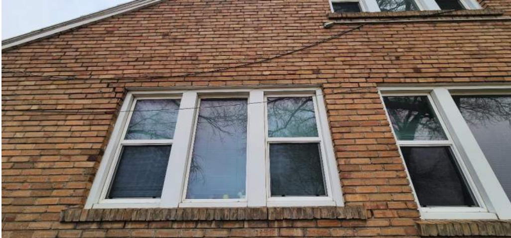
Windows have been retrofit with dual-pane vinyl and cased with aluminum trims. Sill brick at several locations is broken or deteriorated. Sealant needs replaced at various locations as well.
