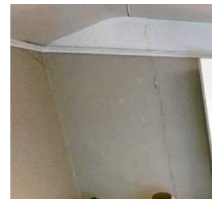
Visible cracks on walls
