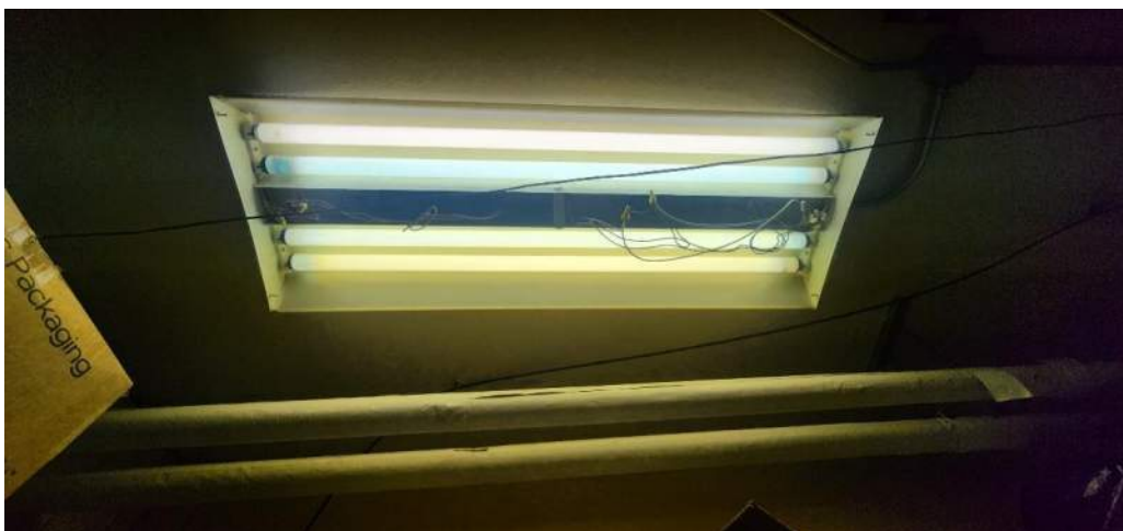
Lighting has been retrofitted at some point in time, this is evident by the amount of surface conduits visible. In some instances, light fixtures remain open and wires exposed, a violation of the National Electric Code.
