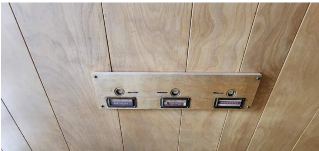
Existing call buttons that are not in use can be removed or upgraded.
