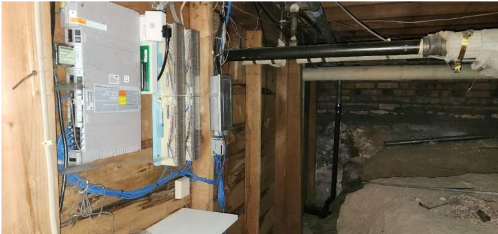
An older phone system and punch-down panel remain within the crawlspace.
