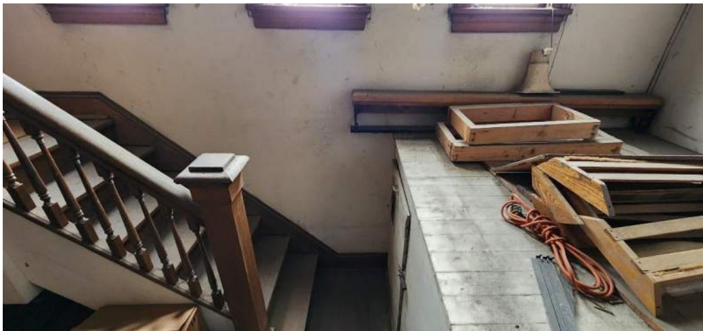
Compressor "room" interrupts landing at lower stair within Belfry. 2024 IBC, Chapter 10 infraction.
