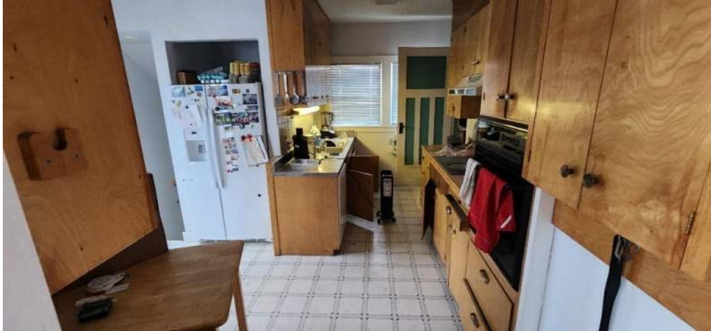
Kitchen is original, cabinets doors were all operable, however drawers show signs of wear. Modernization of the kitchen is recommended. Flooring is aged and shows wear.
