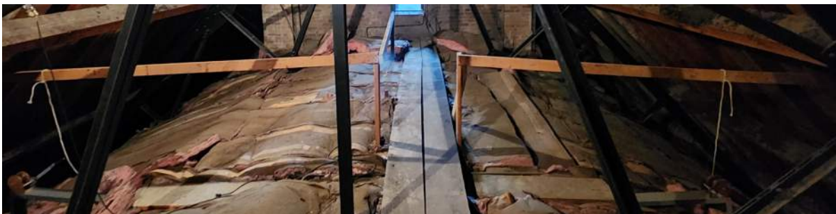
Main catwalk in the Attic lacks OSHA compliant handrails Secondary catwalks to the light cranks lack OSHA compliant platform and handrails
