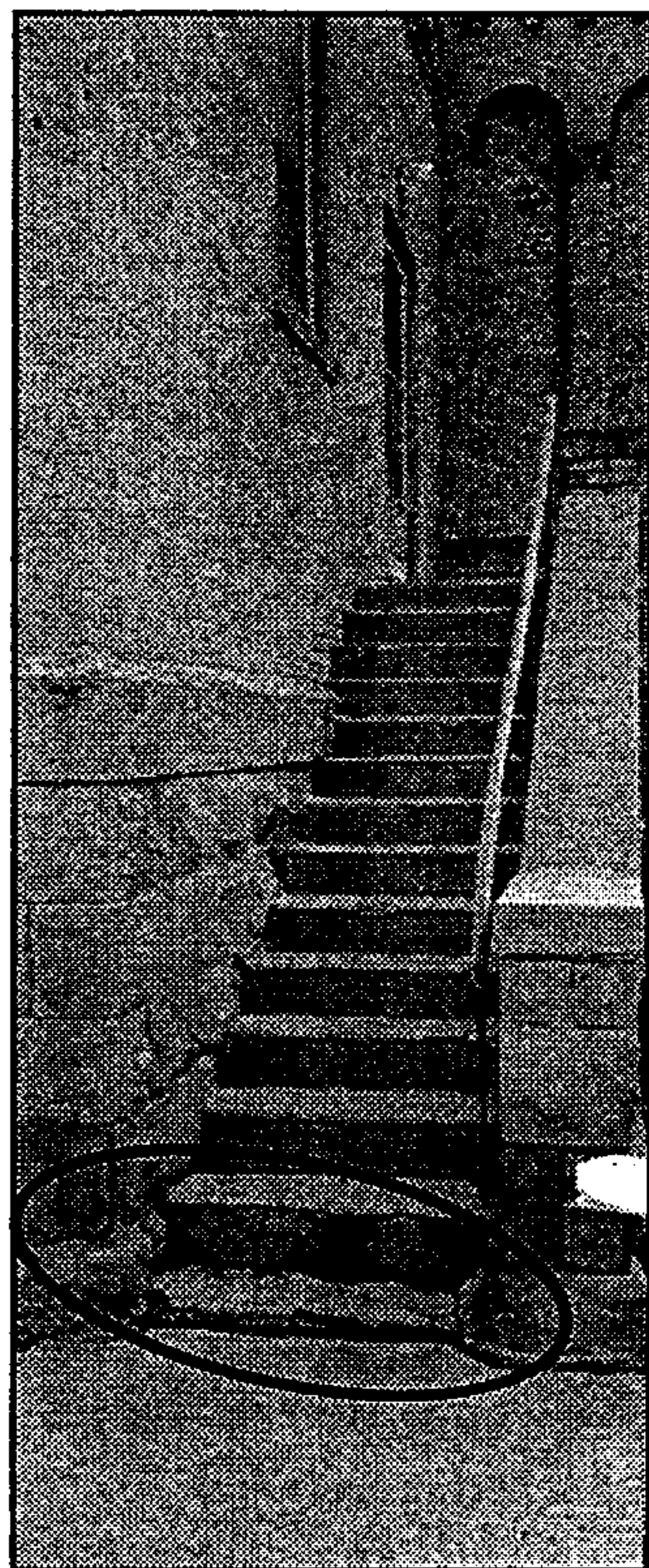
Note: Water damage on landing.
