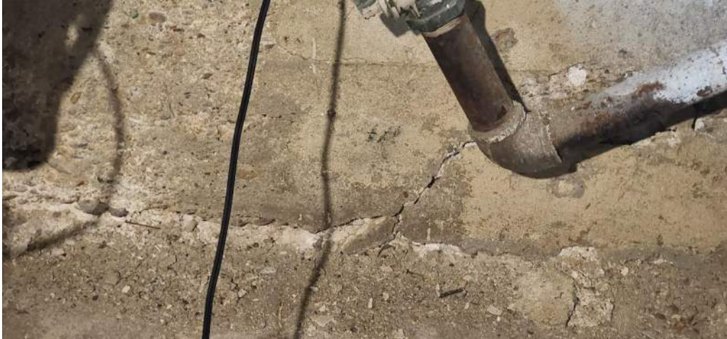
A closeup of the spalling and fractured concrete previously noted. At the floor/wall intersect, is where the concrete shows the most damage. This is the result of long-term moisture influence from leaks, as well as exterior below grade.
