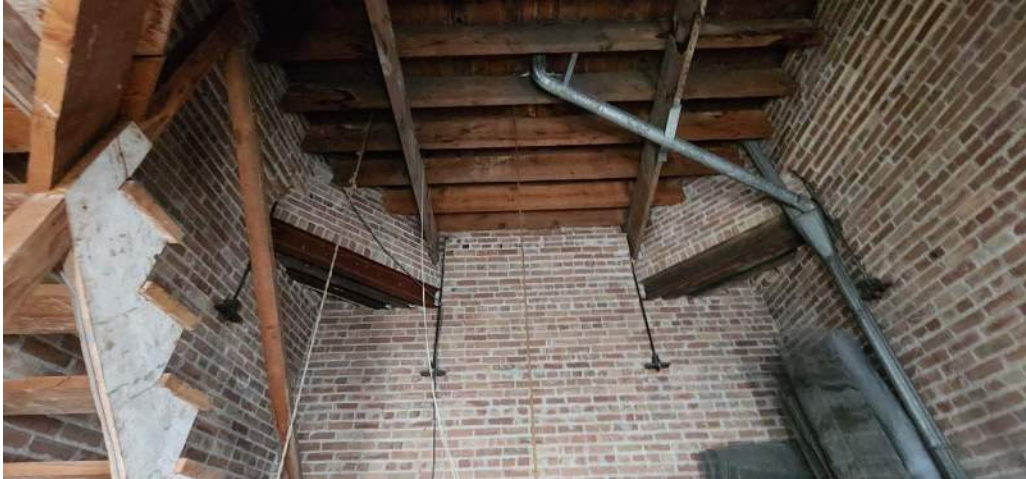
Interior of upper Belfry, masonry appears in good condition. Wood structure shows signs of water damage from previous leaks.
