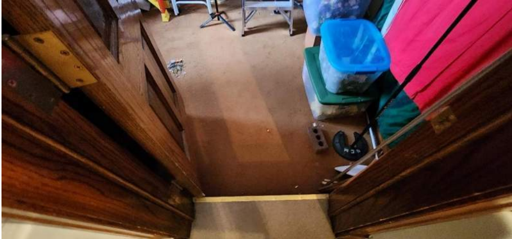
A smaller storage room exists off the Altar, also with a step in the doorway and lack of landing.
