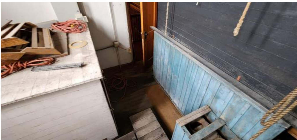
Door to Attic & Belfry cannot open due to construction of organ.
