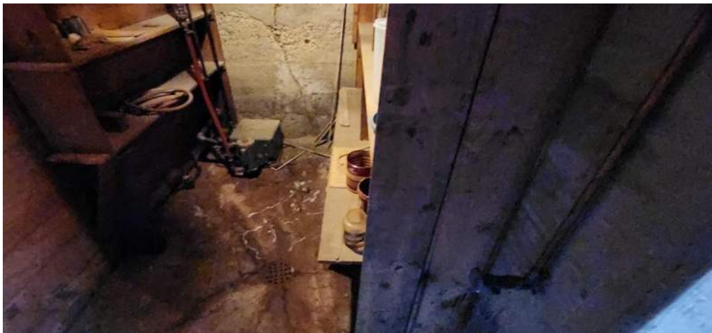
Floor drains are present in slab as well, helping minimize the overall damage from moisture entering through various penetrations in the wall.
