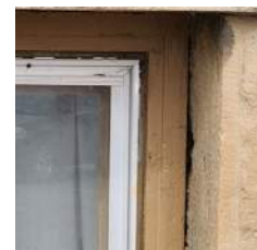
Void around casing
