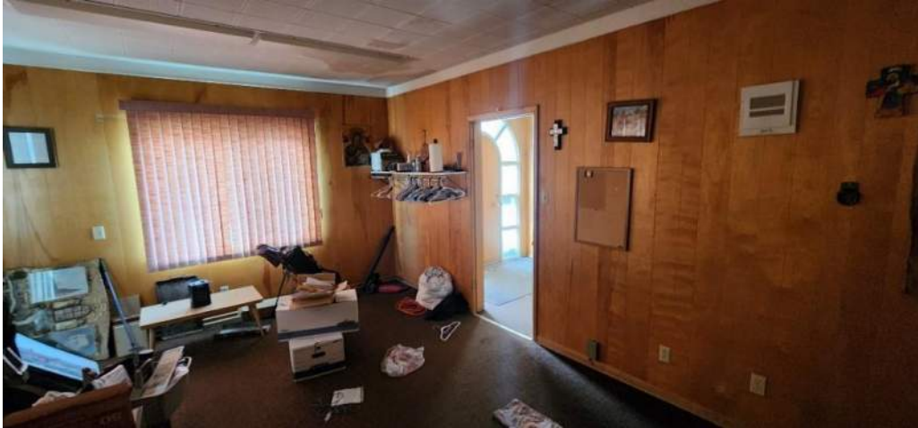
Some signs of previous water leaks from the floor above were visible.
