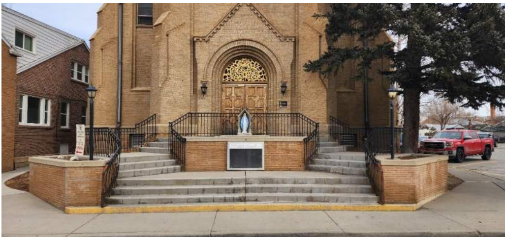
The stairs at the main entry lack handrail extensions and an intermediate rail on the lower section. The lower section also steps directly into the public right-of-way and has been painted yellow as it is outside and beyond the handrails that do exist. To provide proper rail extensions, would require reconfiguration and reconstruction of a majority of the stairs and planters.
