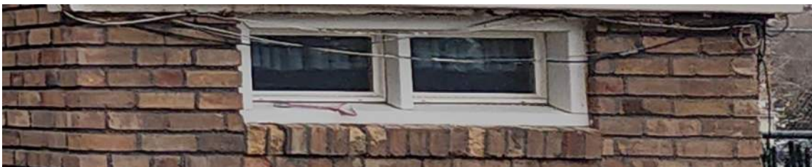
Severely worn sill brick under window – significant weathering of mortar visible
