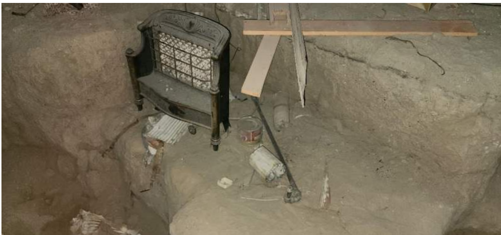
An old gas heater was visible in the crawlspace, no lines are active to the unit as it is out of service.
