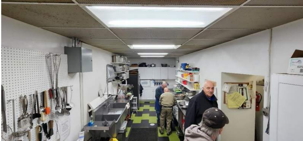
The ceiling within the kitchen appears aged and in need of cleaning/replacement.
