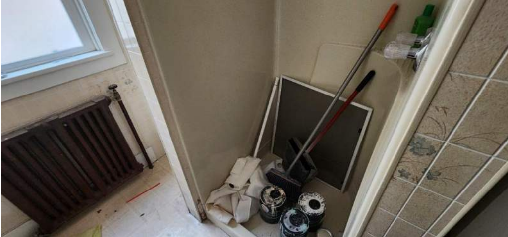
Bathroom has FRP instead of tiling. The FRP is dated and various termination/transition strips are showing signs of failure.
