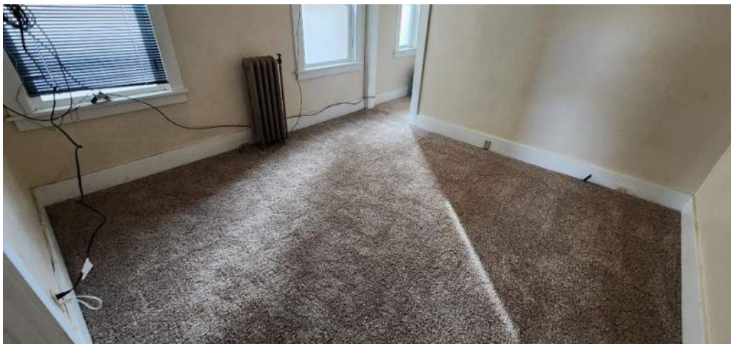
Carpet was clean and taut. An outlet has been added in the baseboard, inconsistent with other outlets in the room.
