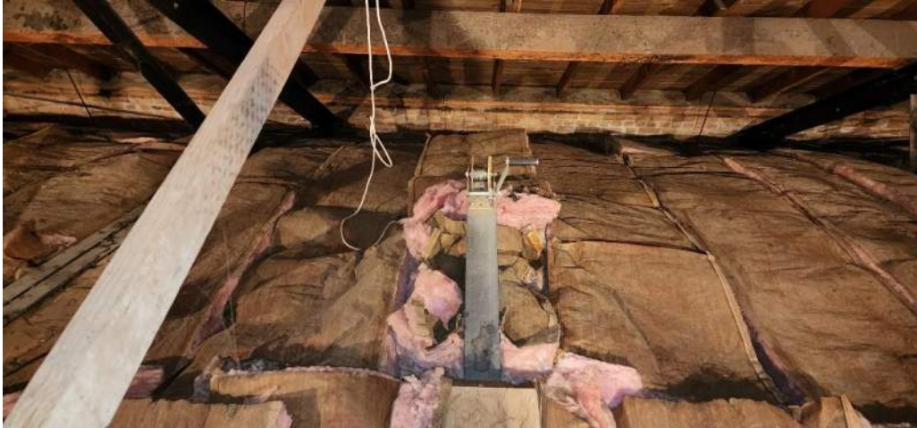
Access walks to lighting cranks do not meet osha. Platform should be widened with proper handrails.
