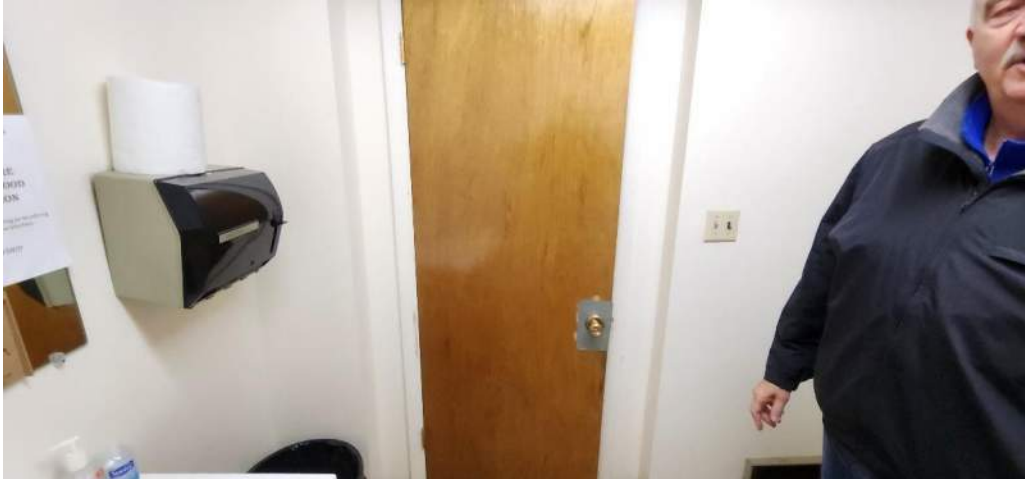
Doors are narrow and limit access to more able bodied individuals.
