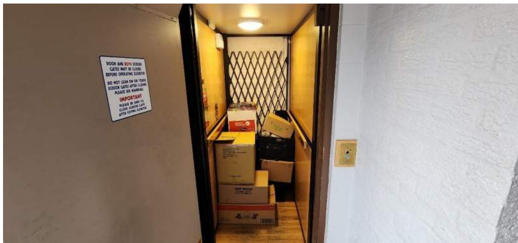
The dimension of the car is restricted to the width of the door and does not comply with the current 48" minimum cab width of a LULA. Accessible space at the door is not present.
