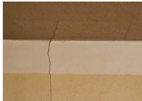
Cracks transferring from wall to ceiling
