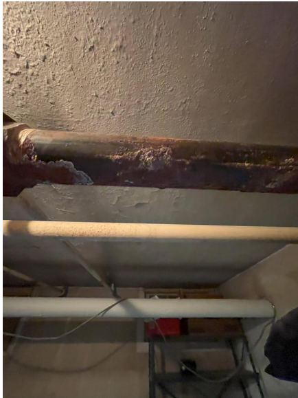
Basement Steam Piping with Pitting and Corrosion
