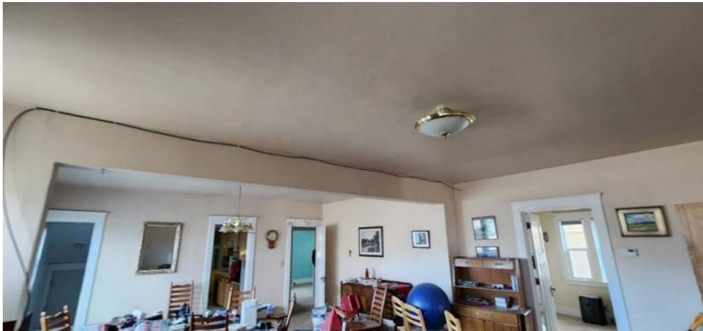
Coax cabling has been anchored to the wall and routed exposed within the room.
