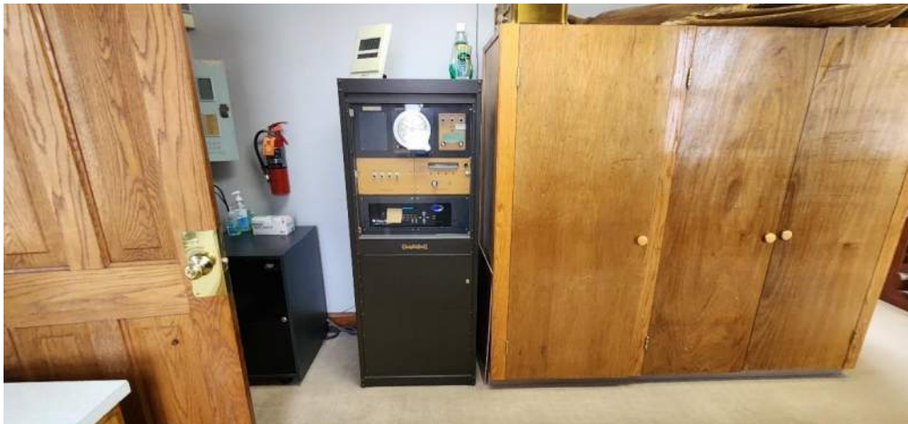
The Sacristy contains plumbing and electronics for music and bells. The space appears to be in overall good condition.
