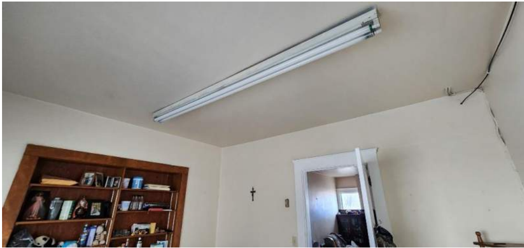
Lighting is aged and should be replaced/upgraded.
