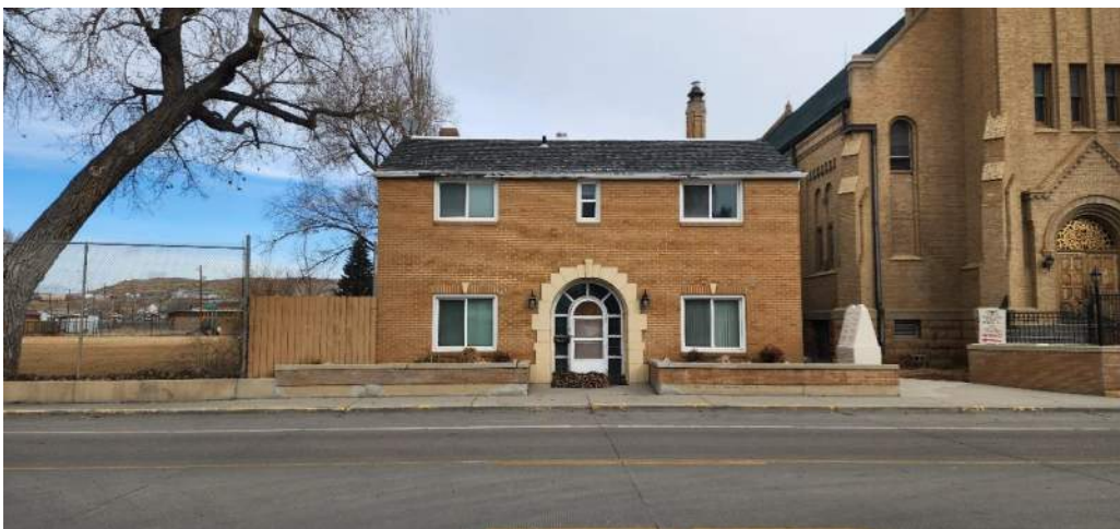
Some settling has occurred at the front, brick repointing and repair is necessary. The finish on the gutters is also failing and peeling. Gutters should be replaced with new.
