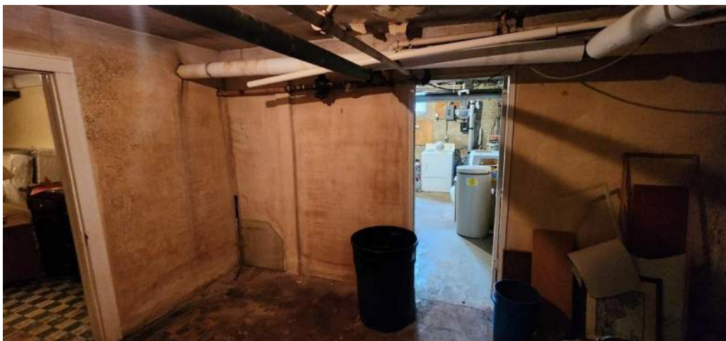
Various rooms have had repairs to ceilings or other patches made. Some rooms have flooring while others are painted or exposed concrete.
