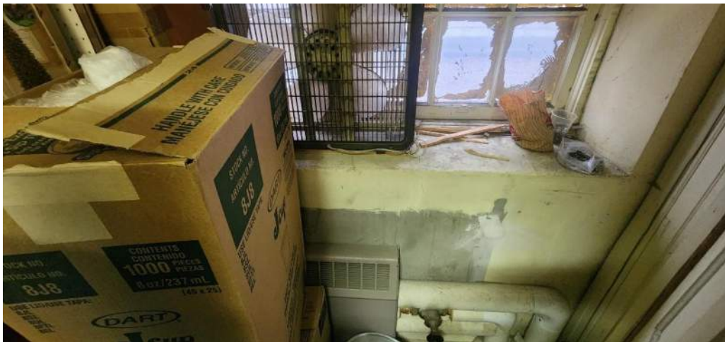
The basement is cast concrete and remains in good shape. Basement windows are single pane and lack efficiency or compliance with modern codes.
