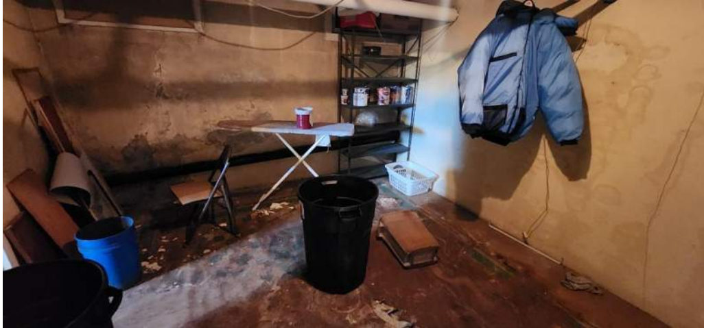
The basement is divided into several rooms for storage or other uses. Framed walls also show significant moisture staining.
