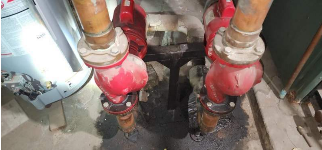
Circulation pumps for the heating system appear to have leaked, oil residue is present on the coupling and the ground around the units.
