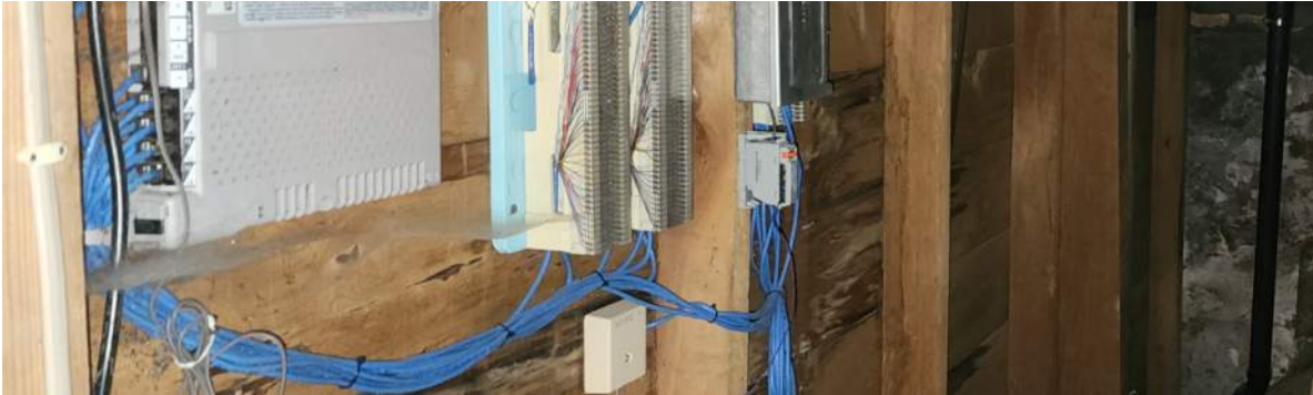
Staining on wood planks and efflorescence on the foundation wall are visible
