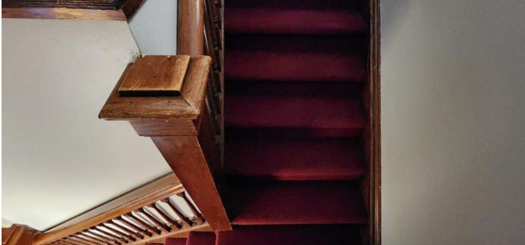
Stair width is reduced due to the handrail and is non-compliant as a result. Adding a second rail would further hinder compliance.
