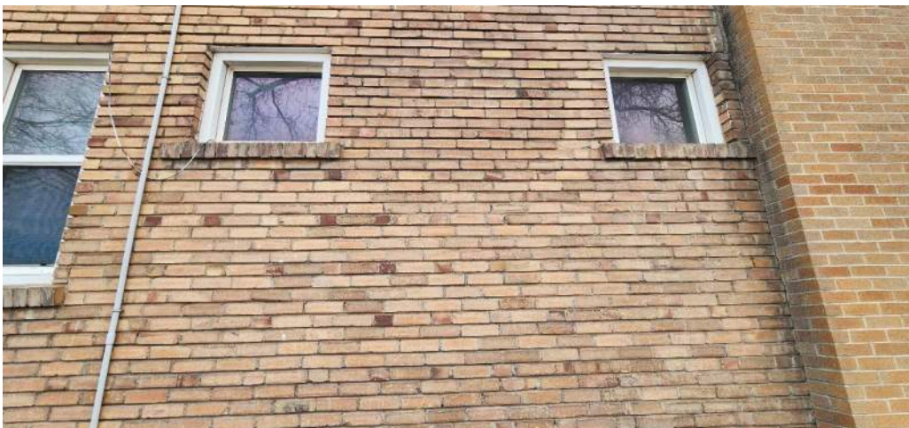
Windows have been upgraded and flashed. The joint between the original Rectory and its addition does not have a control joint, brick is butted together. This should have a flexible joint with sealant. Several bricks show significant moisture damage and staining at this joint.
