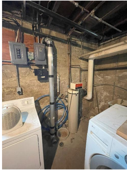
Water Softener and Domestic Copper Piping
