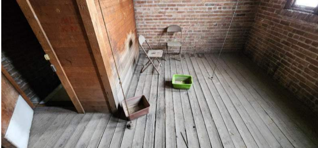
Floor of upper Belfry is curled from moisture infiltration. Structure remains sound, but shows sign of excessive drying.
