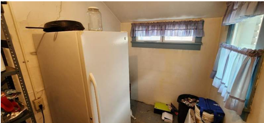
Utilities have been expanded in the basement with upgraded electrical at some point. Behind the fridge and as low as the outlet, more cracking and spalling in the wall are visible.
