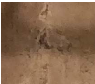
Spalling impacting finish coat
