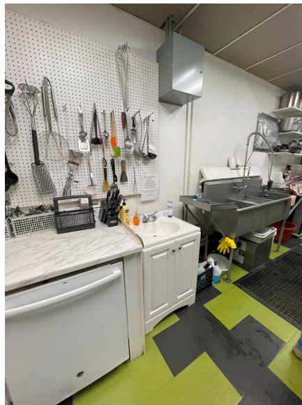
Handwash Sink and Triple Compartment Sink
