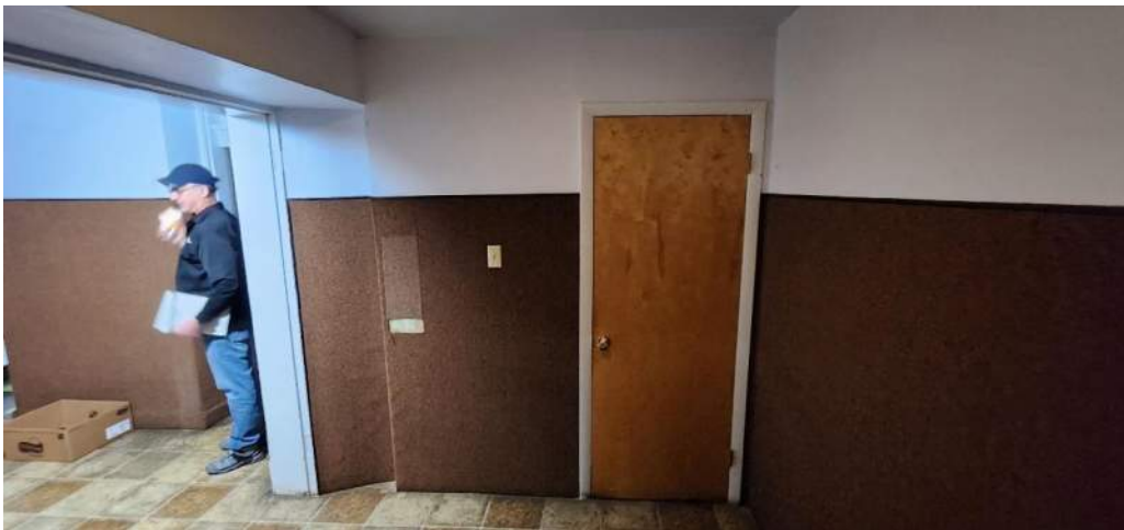
Many of the doors within the space are not 36" wide, thus are not barrier free compliant.
