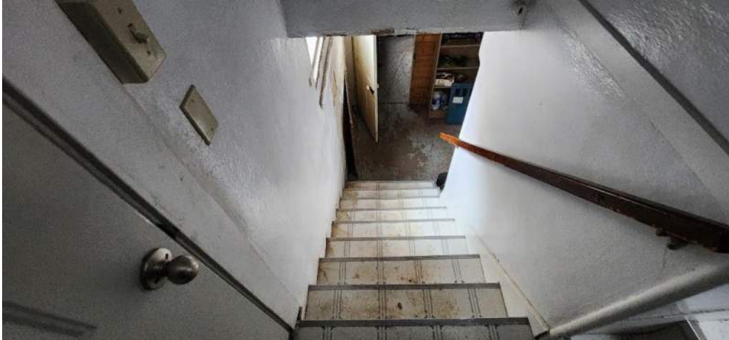
Flooring to the basement is significantly worn and should be replaced.
