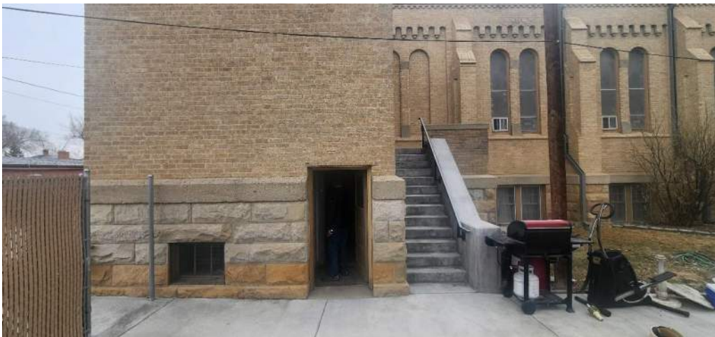
The stone base appears to be in good shape around the exterior. Brick requires repointing at a number of locations.
