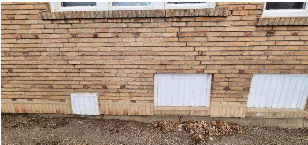
Various windows have been filled in at the top of foundation. These are the locations where more moisture damage is present within the basement. Movement can be seen in the mortar lines as well.
