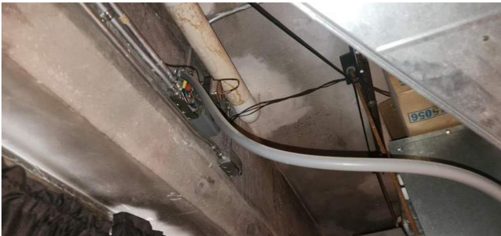
Uncovered junction boxes were visible, this is violation of the National Electric Code.
