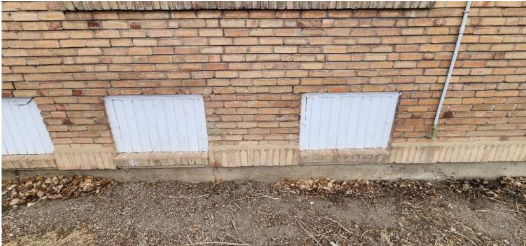
Various windows have been filled in at the top of foundation. These are the locations where more moisture damage is present within the basement. Movement can be seen in the mortar lines as well. At these locations, there is concrete pitting and signs of wear visible above the grade line as well.
