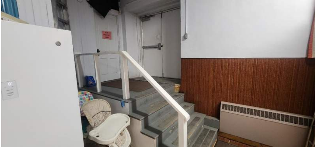
The stair does not have a compliant handrail with extensions and balusters.
