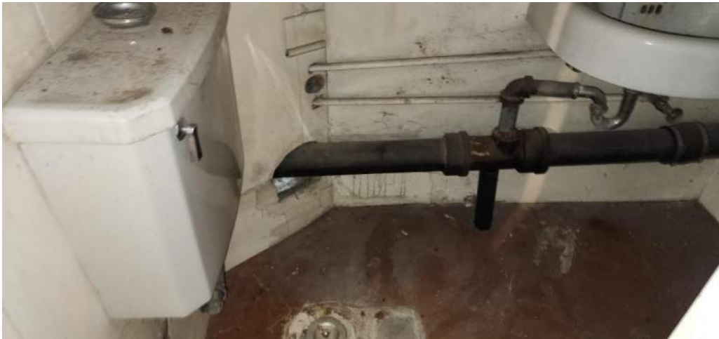
Partial plumbing fixtures remain where a toilet was removed. Only a rubber plug remains at the floor termination. It is unclear why the toilet was abandoned, however, deteriorated plumbing below the floor slab is likely the cause.
