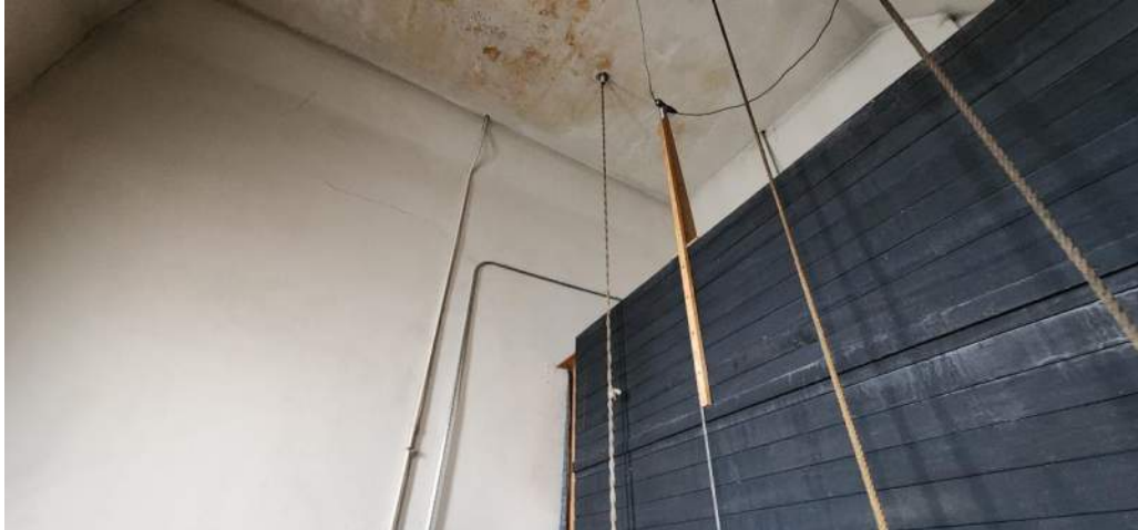
Surface mounted utilities and cables to the bells.
