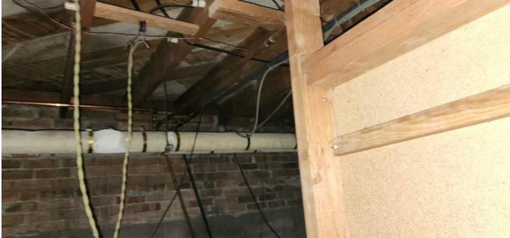
Insulation on plumbing has been patched at various locations. It is not confirmed, however, components of the insulation may contain asbestos.
