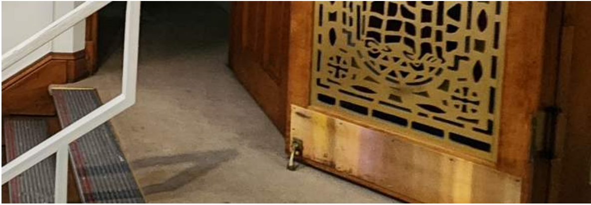
Constrained access to Cry Room and Confessional lack clear floor area of an Accessible Route
