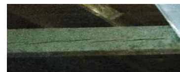
Minor splits on purlins
