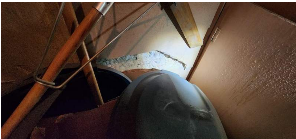
In the storage room near the kitchen, there is evident water damage at the foundation. There was at one time a water line leak that existed for an extended period of time. Damage should be repaired.
