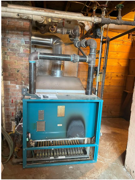
Damaged Boiler- Steam Piping without Insulation
