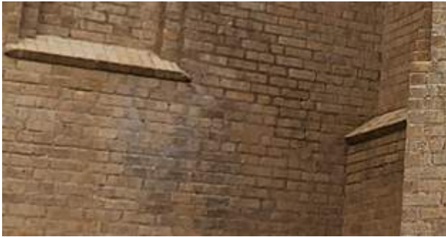
Staining of brick near main entry
