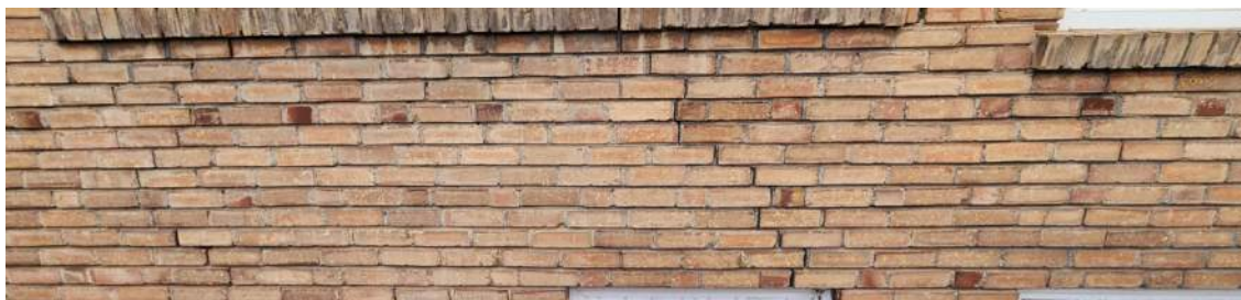
Typical appearance of veneer with separation at mortar joints between openings
