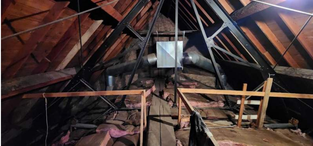
Attic has clear access from one end to the other for servicing. Catwalk width appears to meet 18" OSHA minimum. Handrails are not OSHA compliant. Missing sections, likely are not 200lbs lateral resistant.
