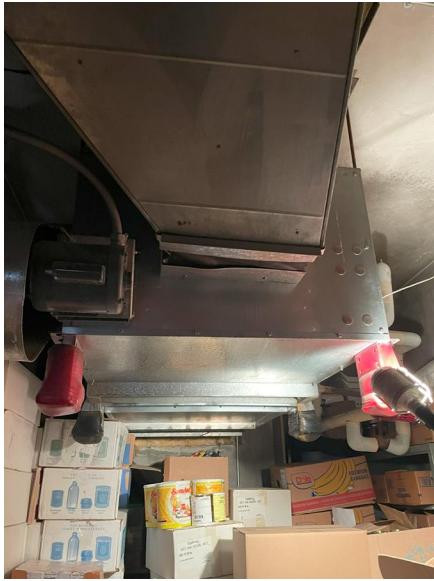
Church Basement Air Handling Unit - back of stage
