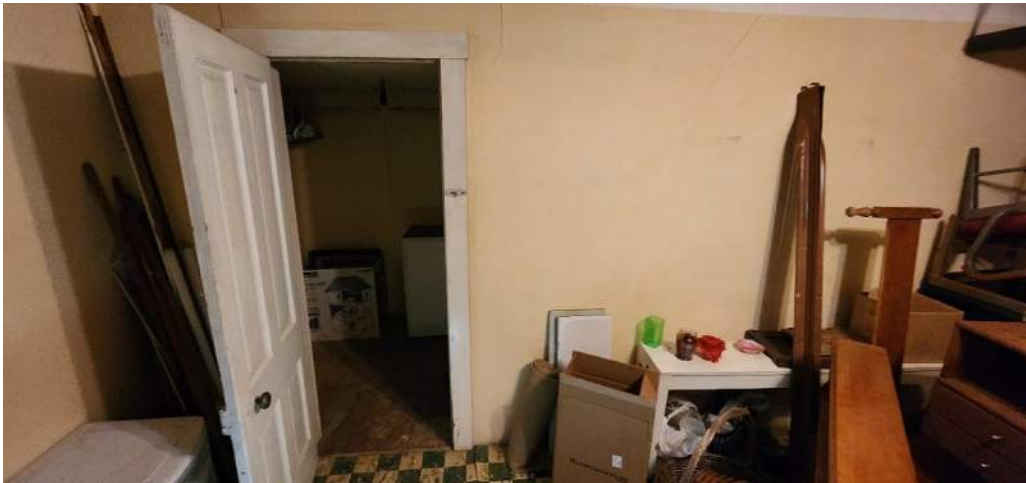
Fractures are visible in a number of framed walls, indicating that the house has settled at some time.
