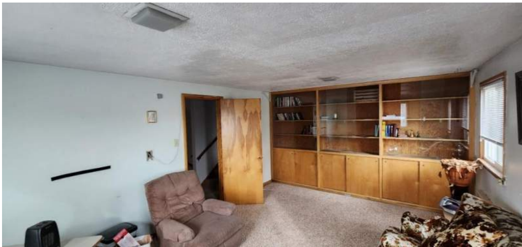
An existing wall box is open with wiring visible. It is unclear the purpose of the wire and needs corrected.
