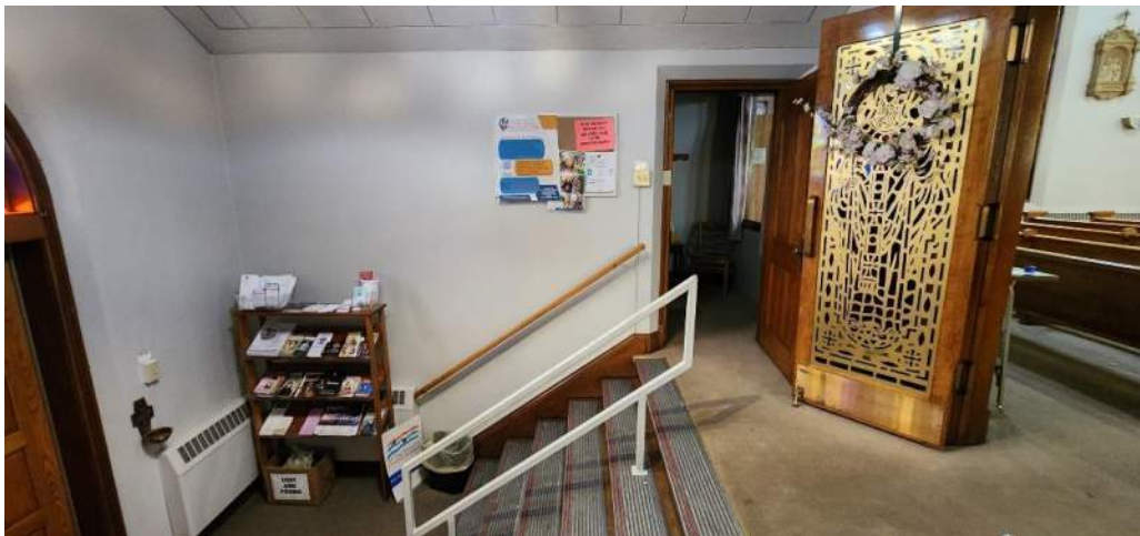
An accessible route for a wheel chair is not present into the Confessional. The door for the room lacks clear floor area on the strike side. The Nave doors disrupt access due to their projection on the landing.
