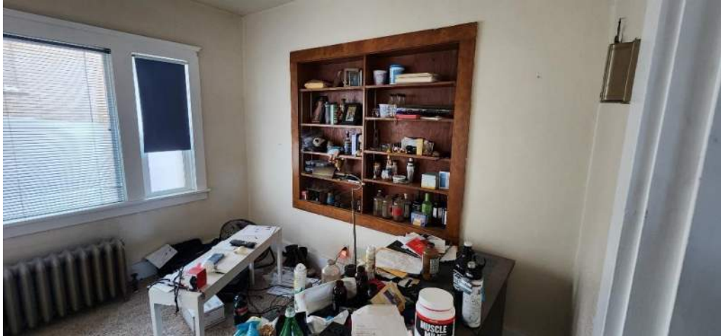
Various styles of window blinds are present in the windows. Abandoned components of the call system exist throughout and should be removed or upgraded.
