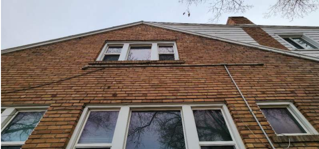
Windows do not stack with parallel jambs, which makes brick prone to movement from floor to floor. Larger mortar gaps are visible between the left hand jambs of the center and upper window.
