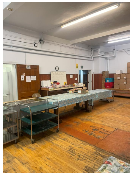
Church basement Heating water distribution piping
