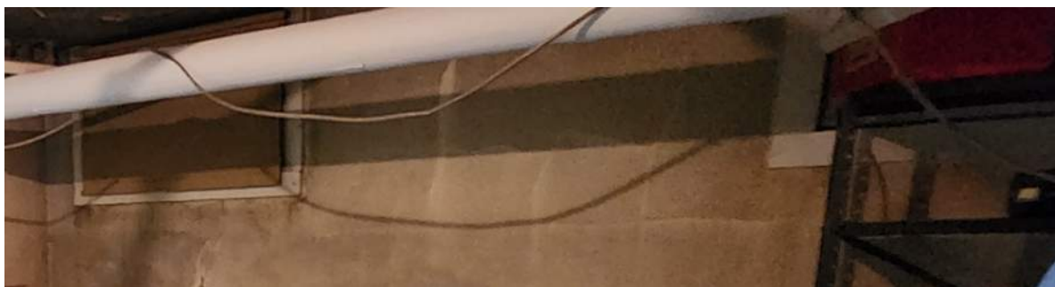
Significant cracking on wall between closed off windows – Openings show signs of historic leaking
