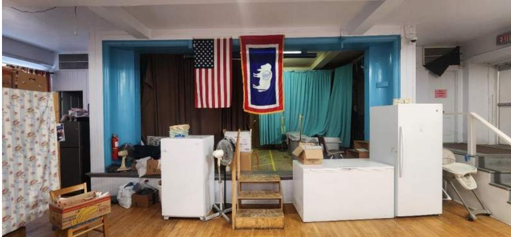
Stage does not have a code compliant access (Stair or Ramp) for users. Currently mostly used for storage.
