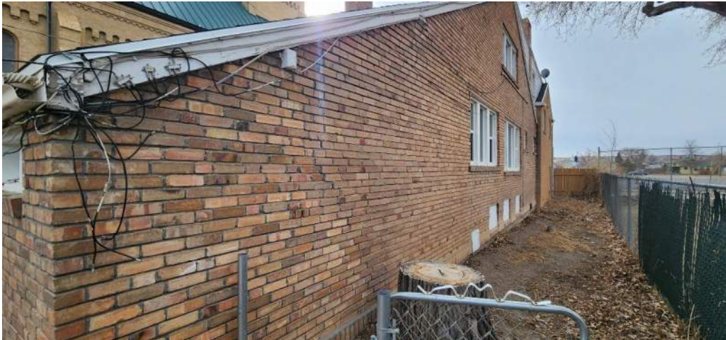
There are a number of settling cracks within the masonry that have gone without repair.
