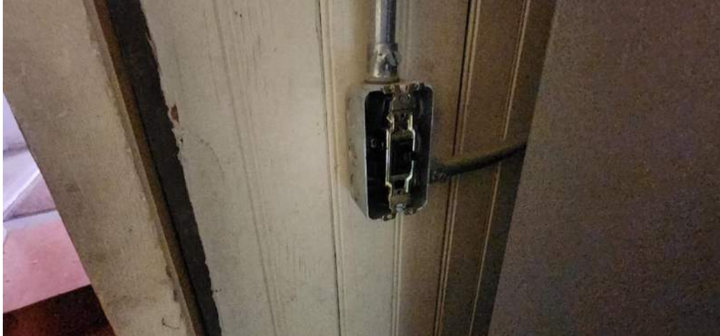
A light switch was missing its cover plate, a violation of the National Electric Code.
