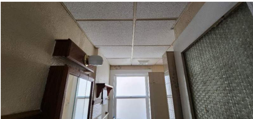
Lighting and fixtures are aged and should be upgraded/replaced. Suspended ceilings in a bathroom require a hardened or scrubbable surface, tiles should be replaced.
