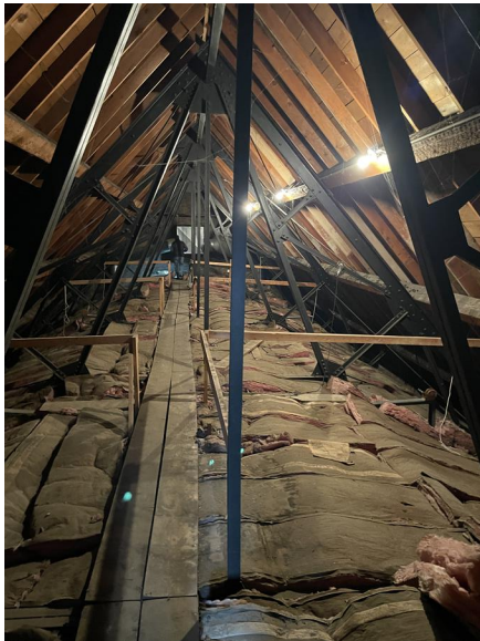
Knob & tube wiring in attic
