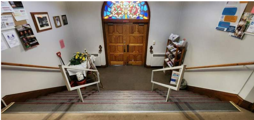
Intermediate handrails at the main entry stairs are present as required. However, all rails present have some form of deficiency for code compliance either in height or extension at the ends. Doors lack egress hardware and rely on manual unlocking for exiting. Daylight is visible through the system, indicating it poor sealing. Repairs have also been made as mating plates are visible on only one of two leaves.
