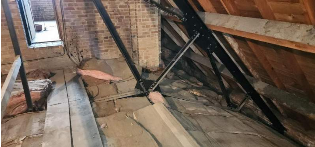
Wood staining from previous moisture infiltration appears dry since the roof replacement and any subsequent repairs were completed. Roof replaced in 1990, repairs/warranty claim made 2010.
