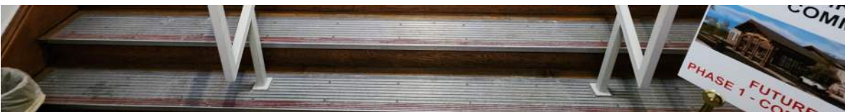
Center handrails do not extend the minimum of 1 tread beyond the lowest tread Center handrails are not rounded at projections and are not round in section
