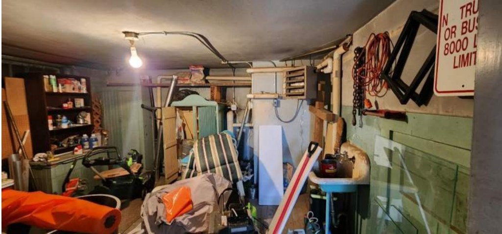
Storage and the main boiler are located in rooms under the sanctuary, accessible from the exterior. The rooms are packed with a number of items from lawn equipment to household goods.
