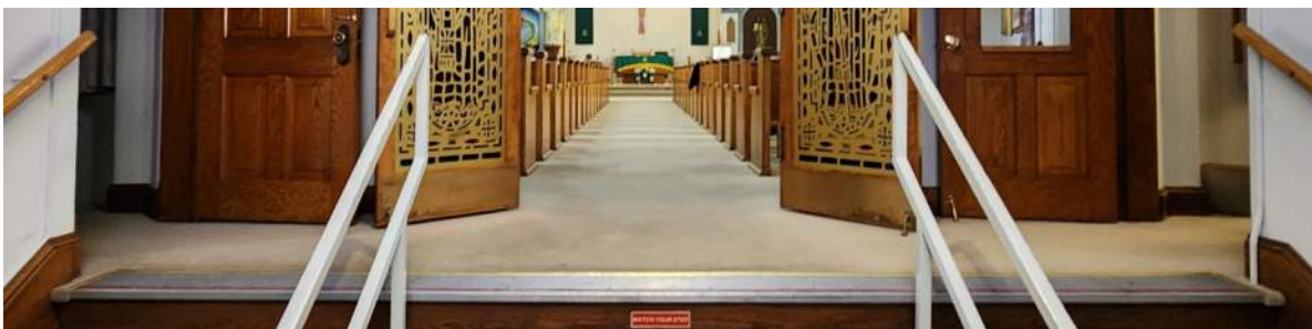
All handrails are short of the required extension (12" minimum from nosing) Center handrails are not rounded at projections and are not round in section
