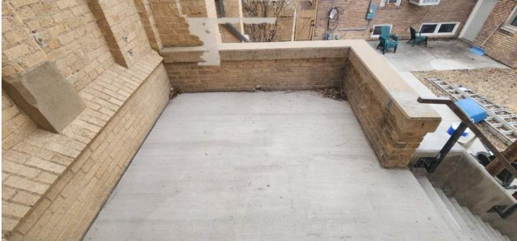
The brick parapet around the landing requires repointing of the mortar and a number of locations.
