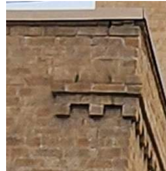
Needed repointing at parapet
