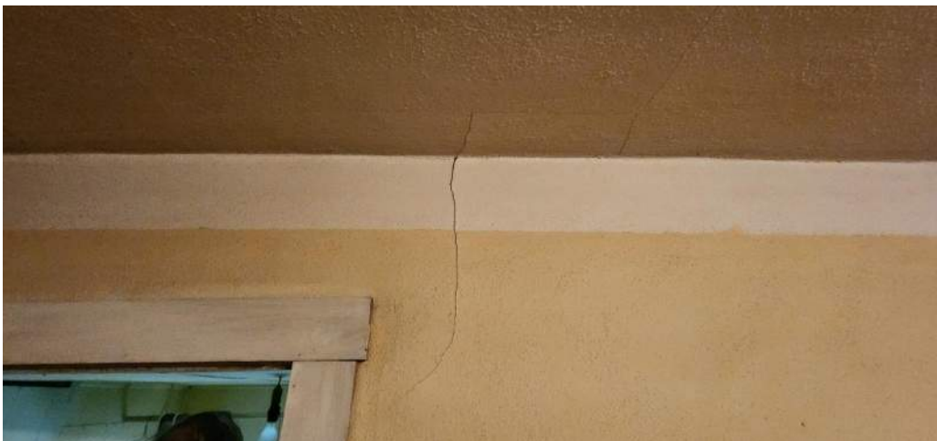
Cracks are not excessive and appear to have stopped. Assuming the foundation condition below grade is confirmed and repairs made to concrete, interior cracks could also be repaired.
