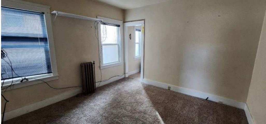
Usual wear from occupancy is visible. Walls require some touch up or patching of small holes.
