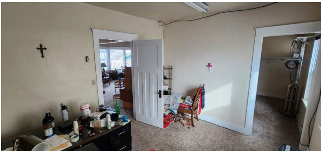
Coax has been added, replaced, and added again. There are a number of cables that are routed throughout various rooms. Some have been painted over, others are newer. Coax can be seen in this room in the corner by the door, along the ceiling, the floor, and in the bedroom.
