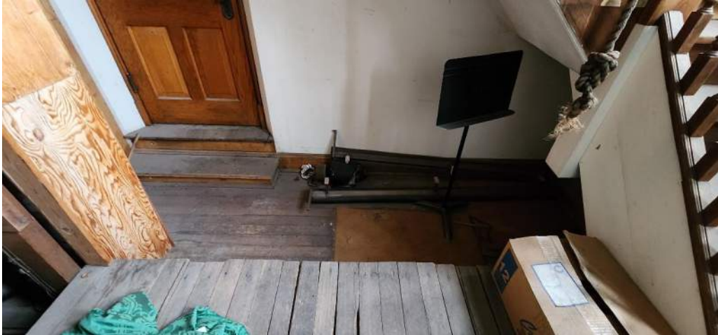
Alternate access to Attic & Belfry – Door swings over steps, inadequate landing area. 2024 IBC, Chapter 10 infraction.
