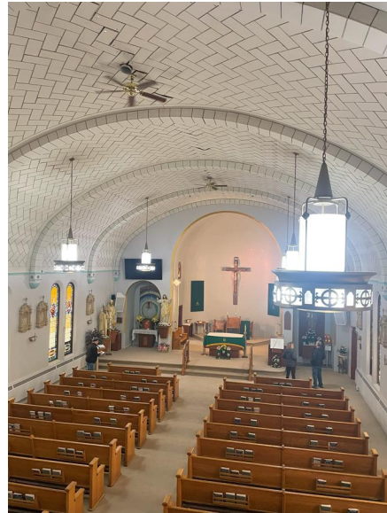
Main Floor Ceiling Fans
