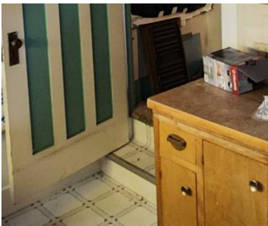
Door lacks landing and handrails
