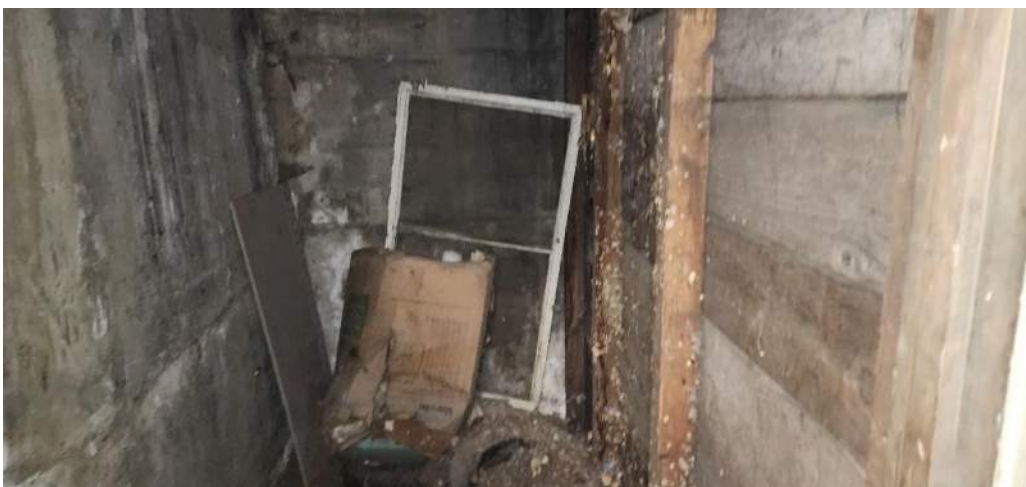
In the deeper areas of the boiler room, trash and other things remain. These items should be cleared and the area cleaned to prevent rodent infestation.
