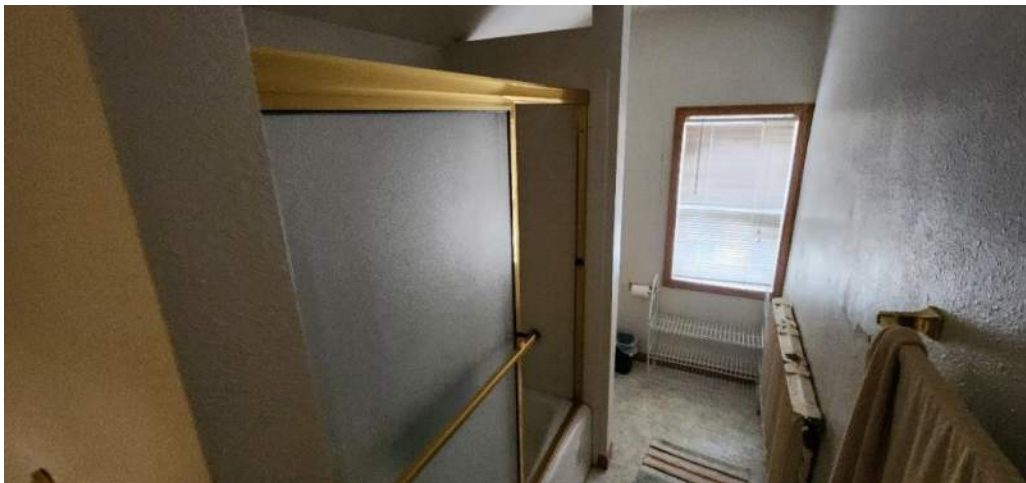
Finishes are dated, sheet flooring in the bathroom did not show significant signs of failure. Paint is peeling above the radiator and some signs of cracking are visible around the window. Finishes should be repaired.
