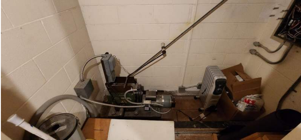
The elevator equipment is aged. It is a cable driven lift system with parts no longer in production. Replacement would require reconstruction of the entire hoistway.
