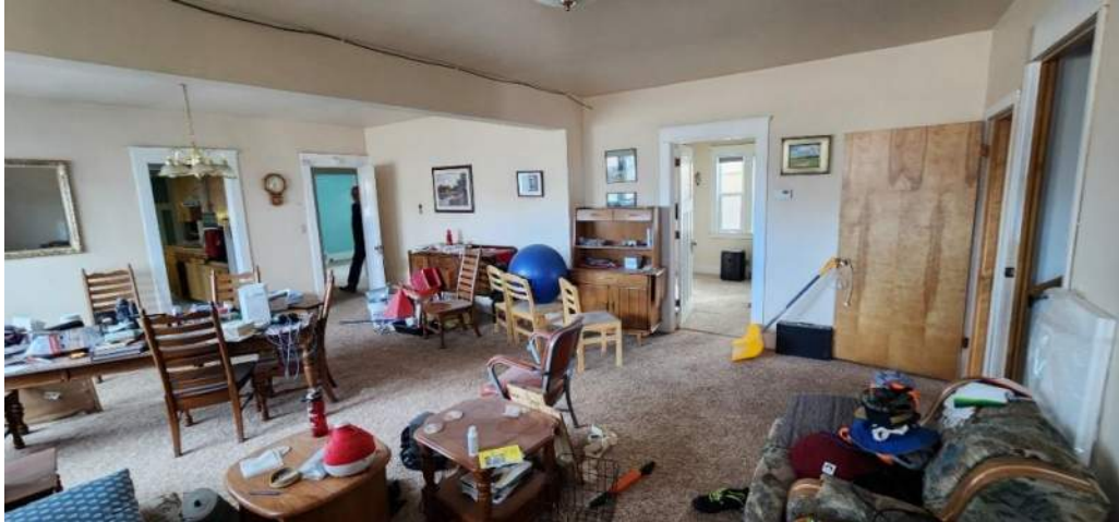
Some signs of carpet stretch were visible in different rooms. This could be resolved by re-stretching where occurs or replacing if desired.
