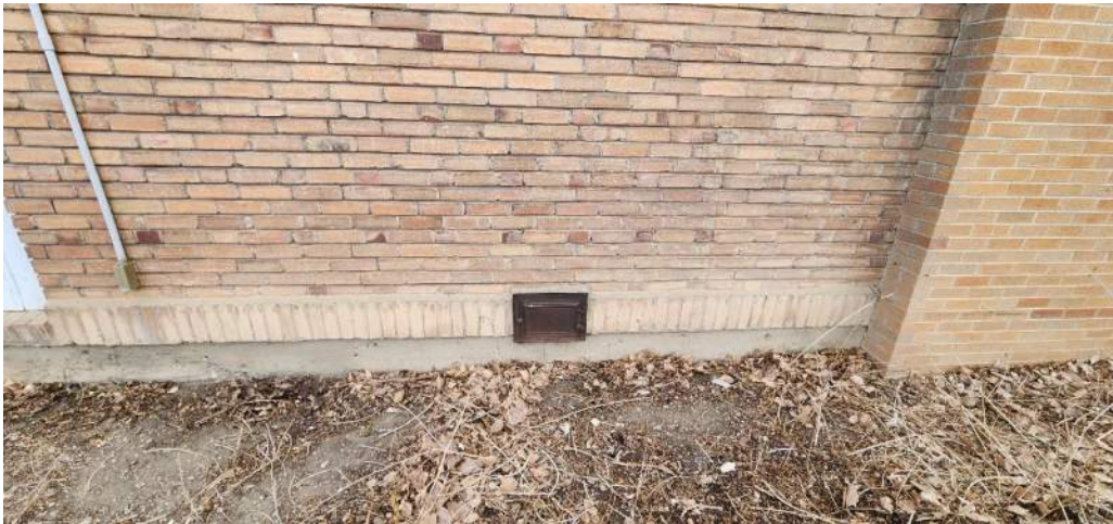
Sill brick at the foundation is in decent condition. Wall brick throughout requires repointing.
