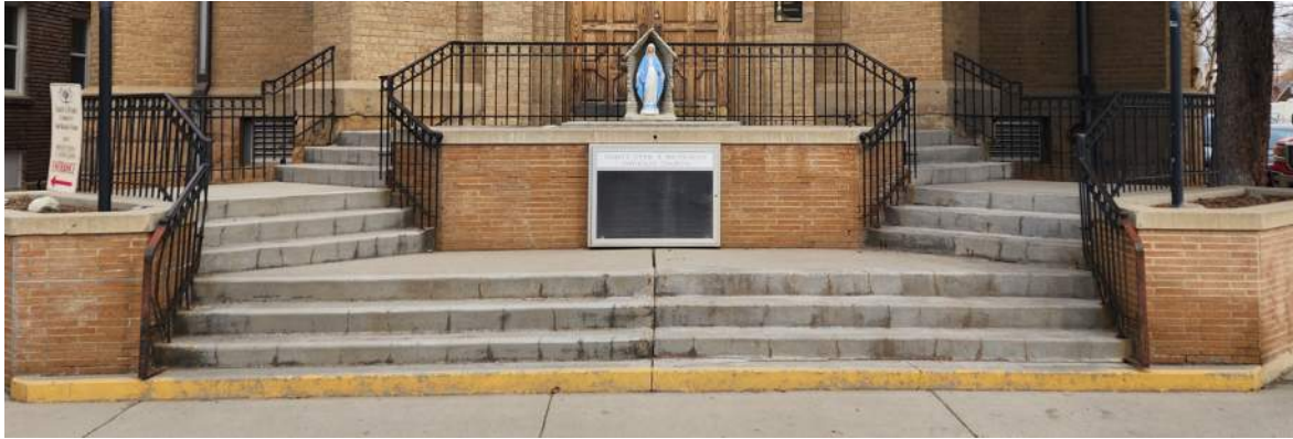
The main stairs lack handrail returns or extensions at various landings.
