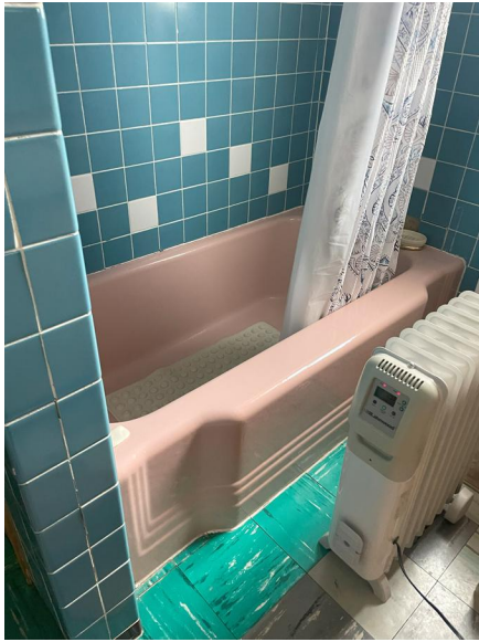
Rectory – Outdated Plumbing Fixtures
