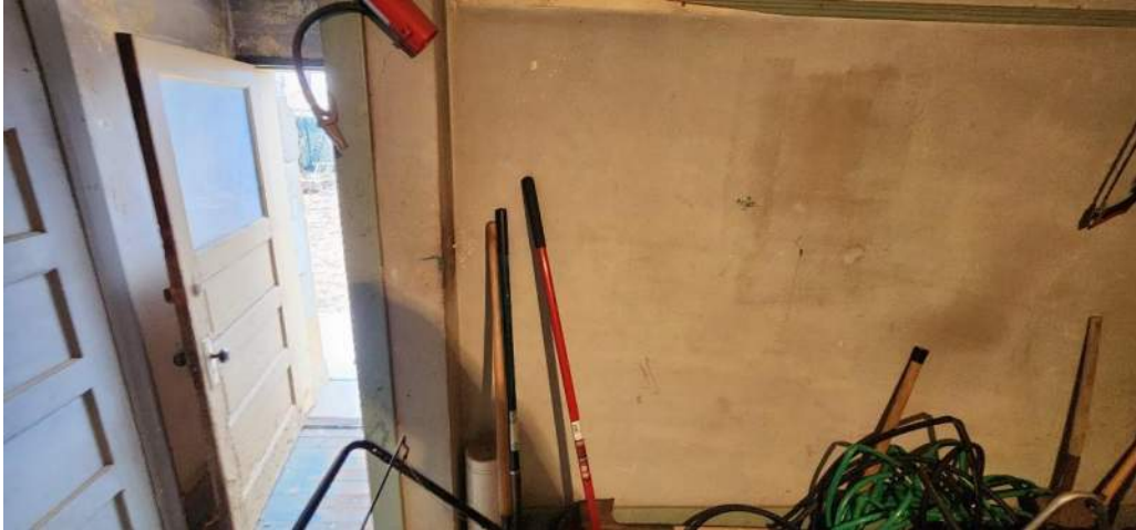
The access to the space is narrow. Creating a challenge for boiler replacement if required.
