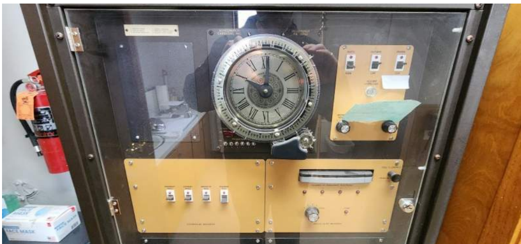
Quadrabell brand electronics for bells remain well maintained and in operation.
