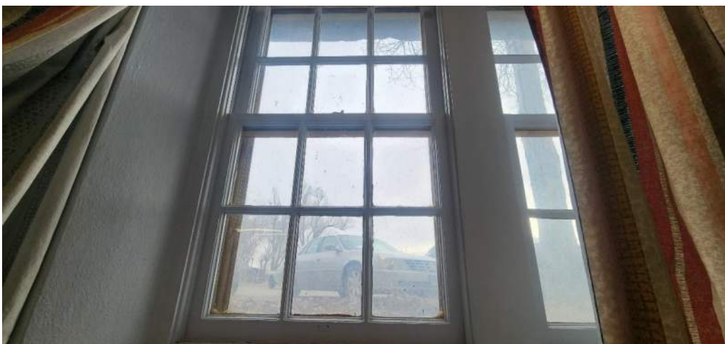
Existing basement windows are single pane and at grade, lacking energy efficiency. They do not meet current efficiency and energy code standards.
