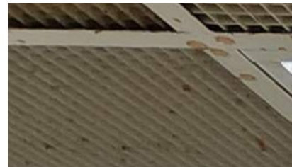
Perf-grid tiles collect grease
