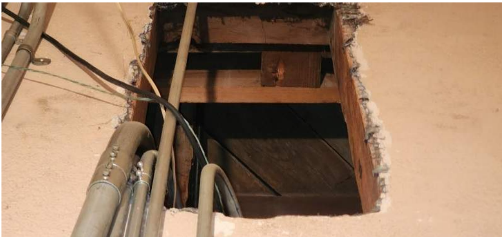
Excessive cut out remains in a storage room for utility upgrades. The wall should be patched back.
