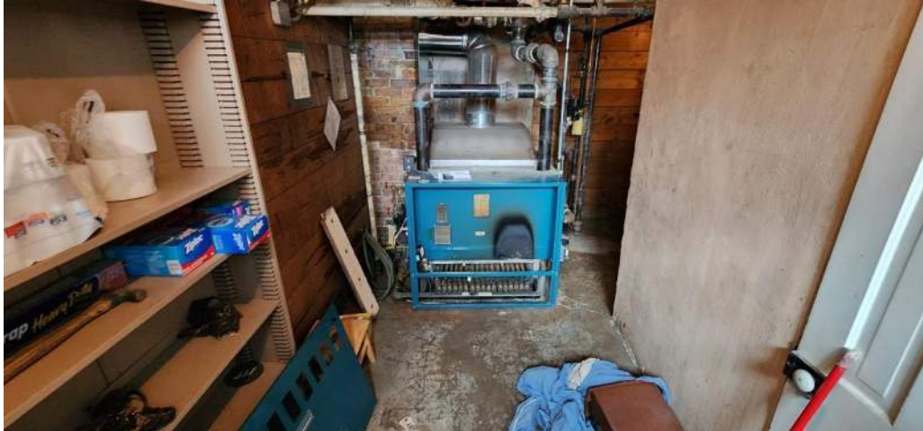
The existing boiler has failed and caught fire. The unit is slated for replacement in the immediate future as it has impacted the heating of the Rectory.
