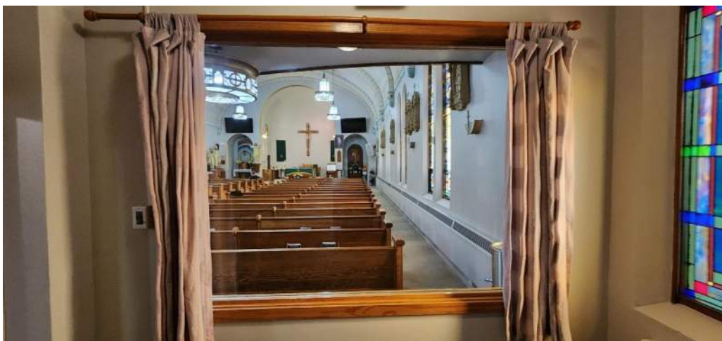
The glazing pane in the cry room is single pane, it could be replaced with a more acoustically private pane design. A dual pane or thicker piece of glazing are both options.
