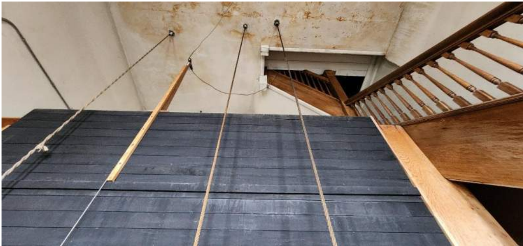
Vertical access to upper Belfry. Handrail is interrupted by floor, headroom is limited. 2024 IBC, Chapter 10 infraction.
