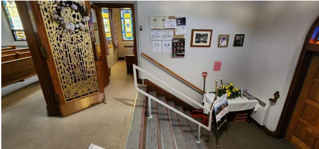
An accessible route for a wheel chair is not present into the Cry Room. The door for the room lacks clear floor area on the strike side. The Nave doors disrupt access due to their projection on the landing.
