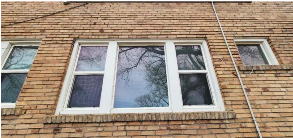
Brick repointing is required in many locations of the Rectory.
