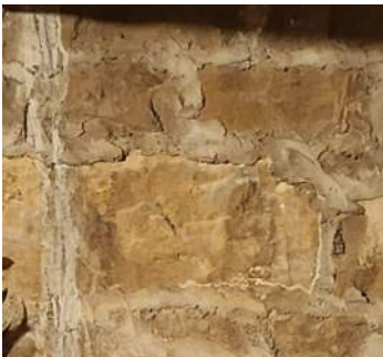
Staining on stone
