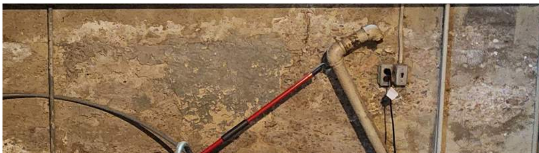
Significant spalling and efflorescence visible across width of room
