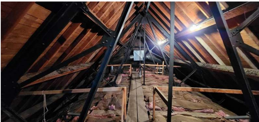
Attic has clear access from one end to the other for servicing. Catwalk width appears to meet 18" OSHA minimum. Handrails are no OSHA compliant. Missing sections, likely are not 200lbs lateral resistant.
