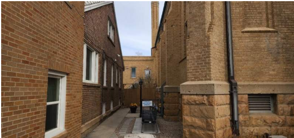
The stone base appears in good shape, the concrete fap has pitted, but does not show structural failure. The brick as mentioned throughout, require repointing in a number of locations.
