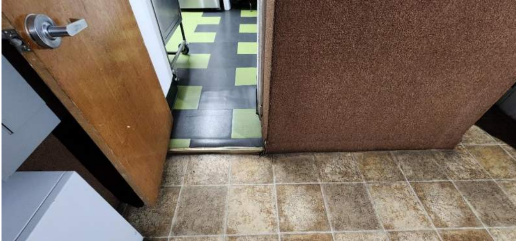
An inconsistent floor transition exists at one of the kitchen entry ways. This is a small hazard when accessing the work space with items in hand and should be corrected to a sloped transition.
