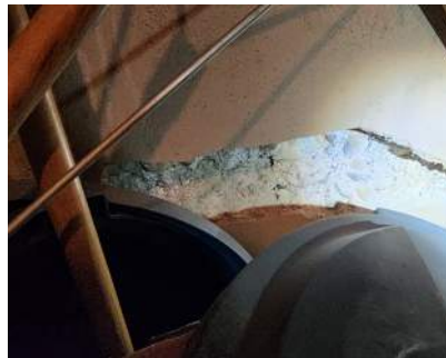
Spalling noted near Kitchen
