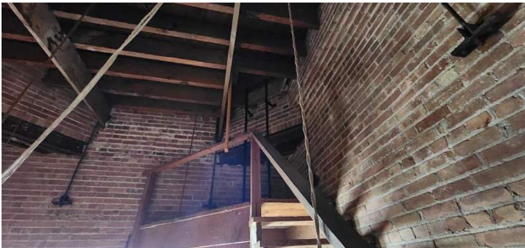
Access to the main bell room above is tight with little landing area to access. Structural connections to the room above remain in tact. Some water staining remains visible on structure from previous moisture infiltration.
