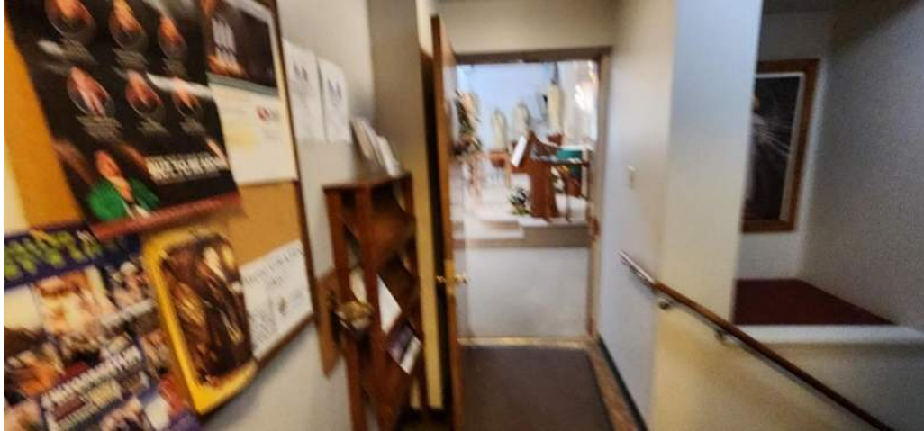
The accessible route from the addition into the church is restricted. Without the door, complies with minimum requirements.
