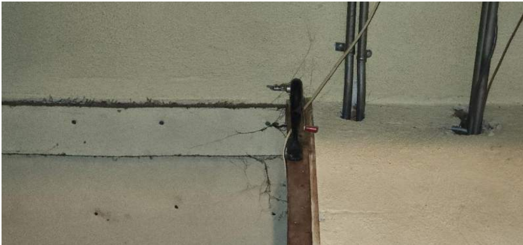
Penetrations through various walls should be patched to improve fire safety characteristics of the walls throughout the basement.
