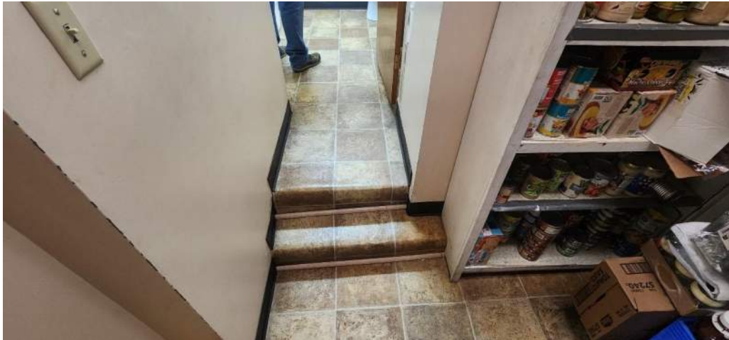
Flooring from the dry storage to the small staff restroom lack handrails, they also are finished in a way that make them non compliant for nosing requirements under Chapter 10 of the 2024 IBC.
