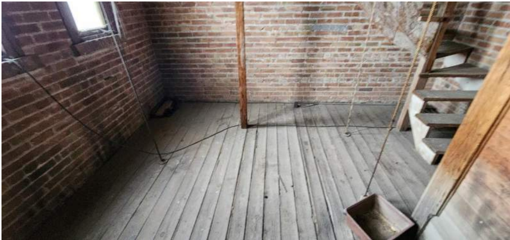
Floor of upper Belfry is curled from moisture infiltration. Structure remains sound, but is also shows sign of excessive drying due to UV.
