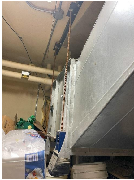
Church Basement Relief/Exhaust Unit -back of stage
