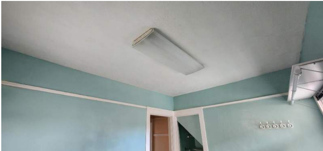
Lighting is aged and should be upgraded/replaced.
