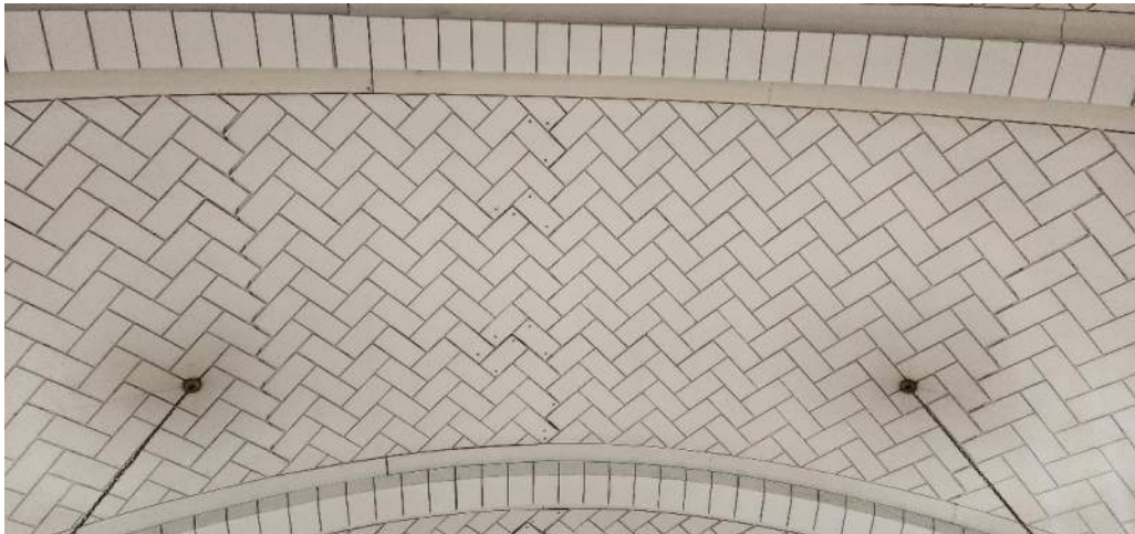
Historically, the roof has leaked. Repairs have been made. Tiles have been resecured to the ceiling along the ridge where necessary. Tiles remain secure, however, could be cosmetically repaired to conceal the past work.
