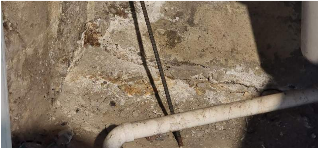
A second closeup of the spalling and fractured concrete previously noted. A random rebar was present leaning in the corner.
