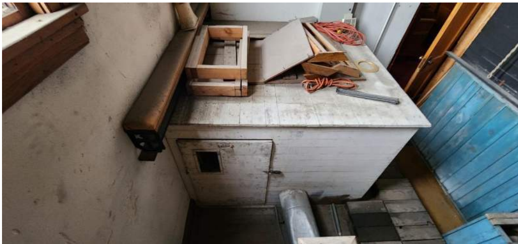
Organ compressor "room" has limited services space and adversely interrupts safe egress.
