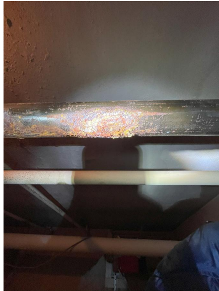
Basement Steam Piping with Pitting
