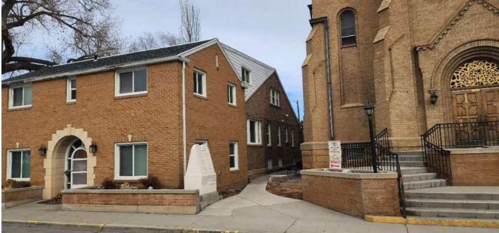
The space between the Rectory and Church is small and allows for moisture runoff of both buildings, and the ground area, to accumulate.
