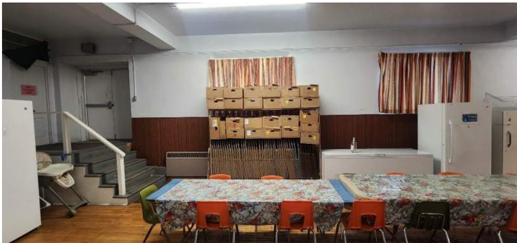
Exterior loading/egress door lacks operation of the second leaf in an emergency. Current codes require both leaves to become active in an emergency. The stair does not have a compliant handrail with extensions and balusters.
