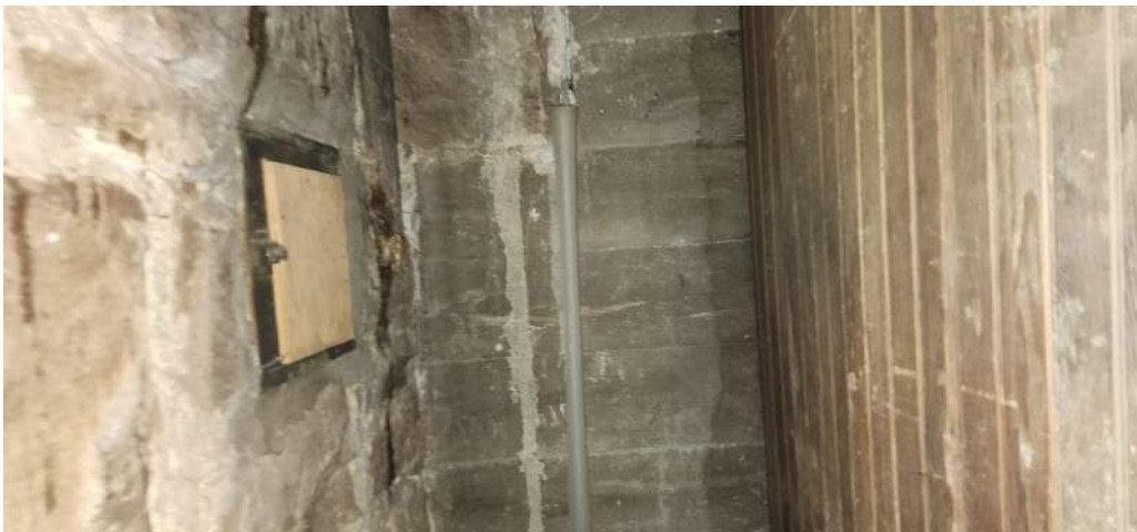
Some staining was also visible on the underside of the concrete landings above.
