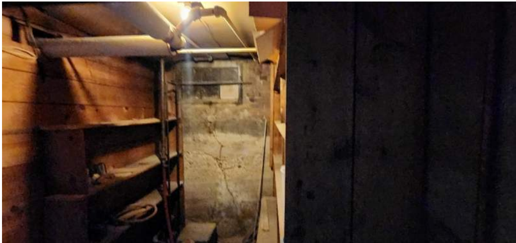
The rectory foundation is concrete below grade. There are several areas where old penetrations in the wall have suffered moisture infiltration and show damages. Movement does not appear excessive and repairs can be made to the visible fractures.
