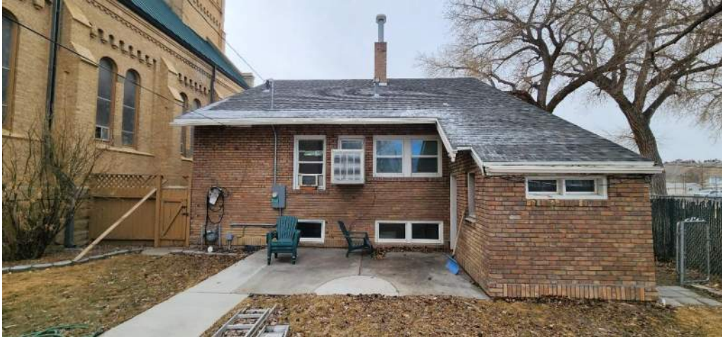
The original rectory is a red brick and is showing age. The mortar is weathered significantly. Sill brick along several windows is excessively deteriorated as well. The shingles have been upgraded in the past, no concern of roof failure noted.
