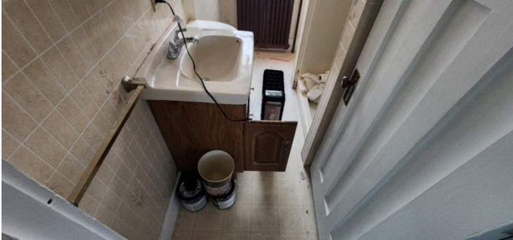
Flooring and fixtures are aged and show wear. Replacement/upgrade should be considered.
