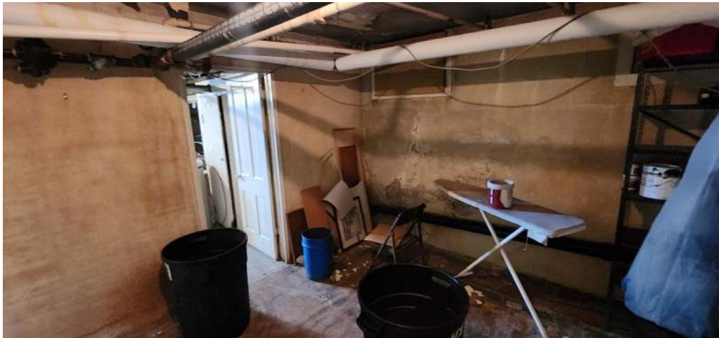
Additional moisture infiltration and damage is noted at another penetration that has been closed off. More spalling of concrete and fractures present.
