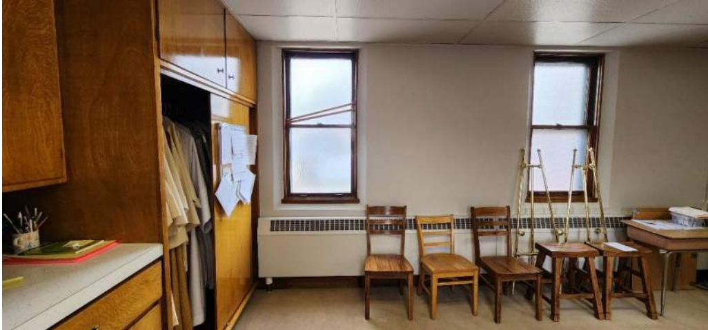
Exterior windows in the church, Sacristy included, do not meet current energy conservation codes.
