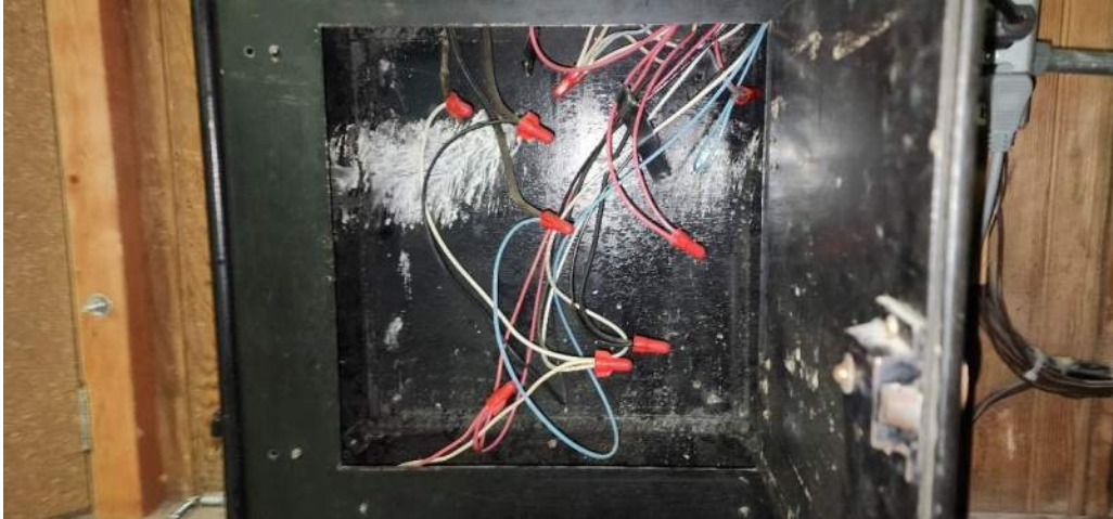
Panels have been converted into junction boxes (see electrical report for additional info)
