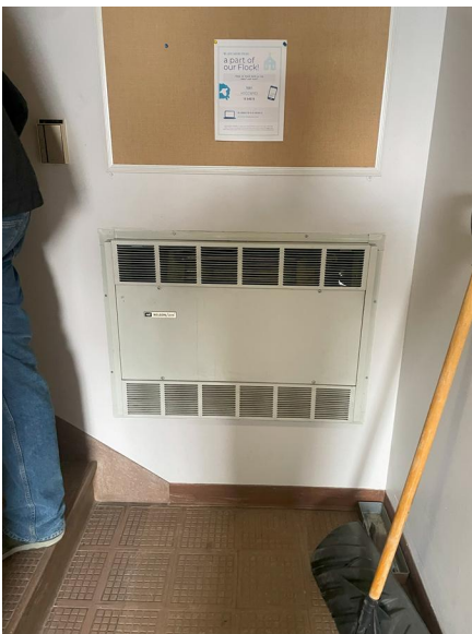
Church basement Cabinet Unit Heater
