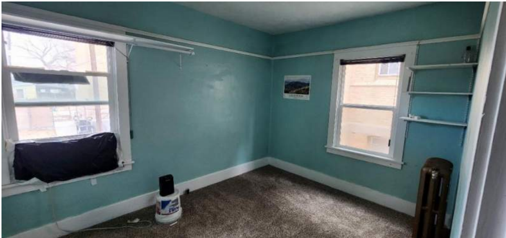
A window AC unit was present in one room and should be removed through winter. Usual wear from occupancy is visible. Walls require some touch up or patching of small holes.
