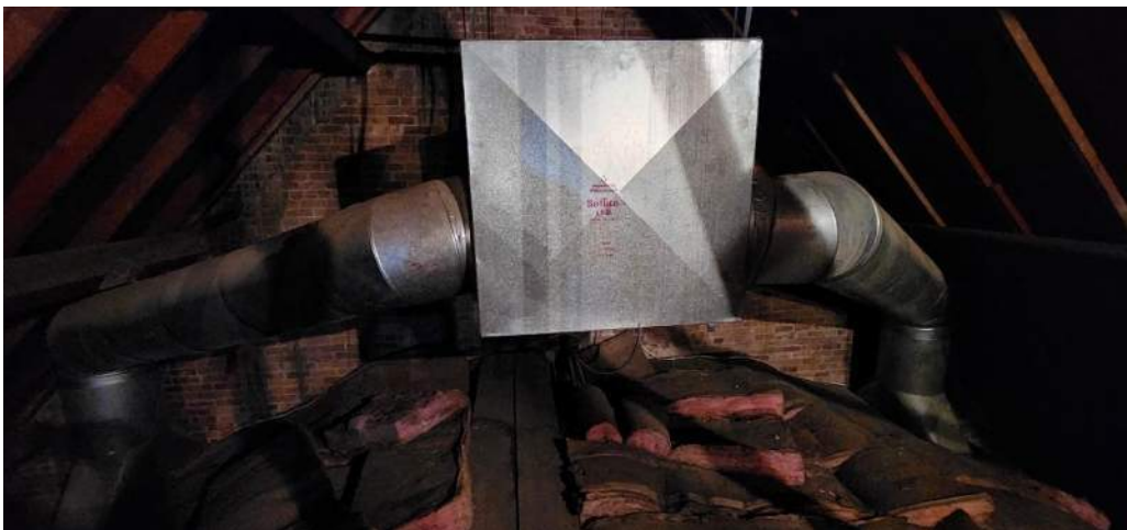
A large mechanical duct is present with round ducts splitting off to feed the Nave below. Any access required beyond or around this unit, does not have compliant platform or rails. Insulation has been placed in a haphazard manner and should be reinstalled neatly.
