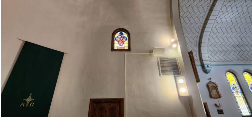
Additional speakers and lighting can be seen installed on wall. Ventilation serving the space has been modified with certain registers blocked off from use. Free air ventilation required by code may be impeded as a result.
