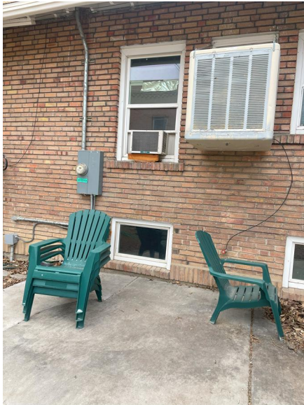
Rectory Window AC and Swamp Cooler
