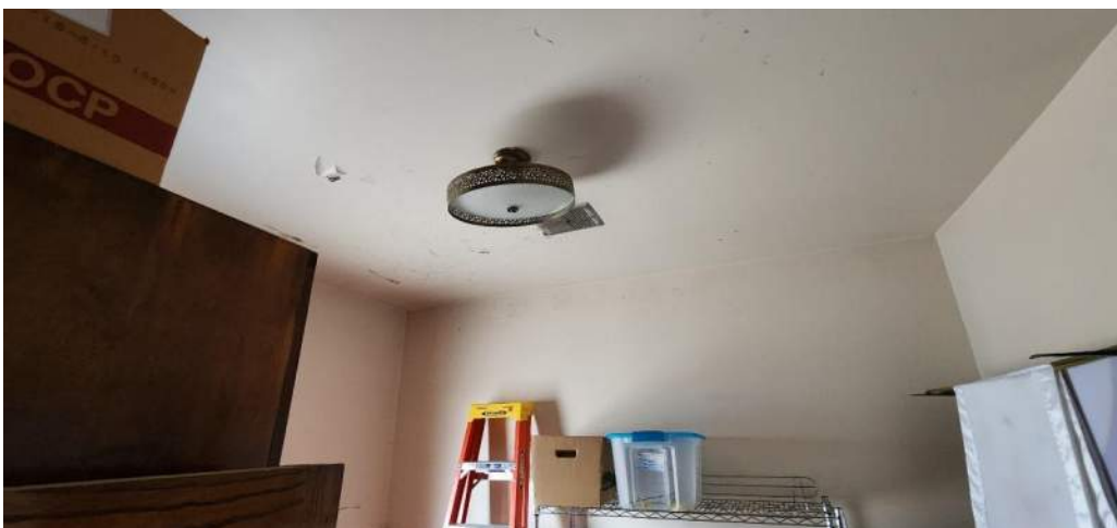
Paint had previously peeled within the space.
