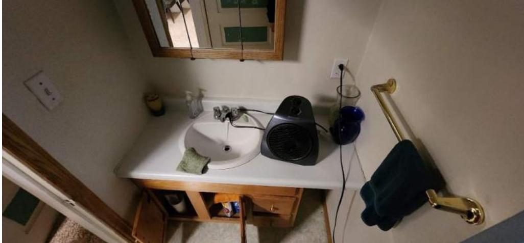
Sealant around fixtures and counters is failing and should be replaced.
