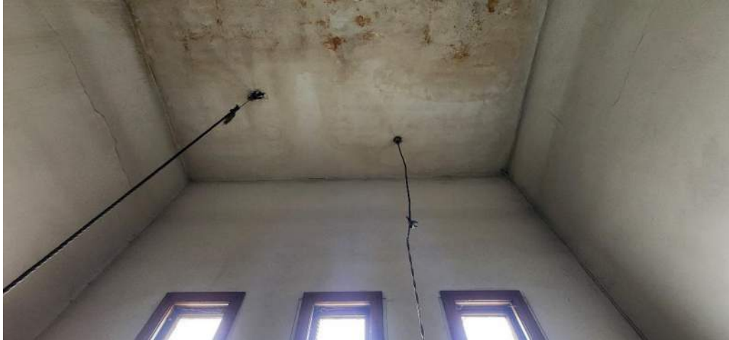
Moisture damage visible, with minor cracking in walls of main Belfry area.
