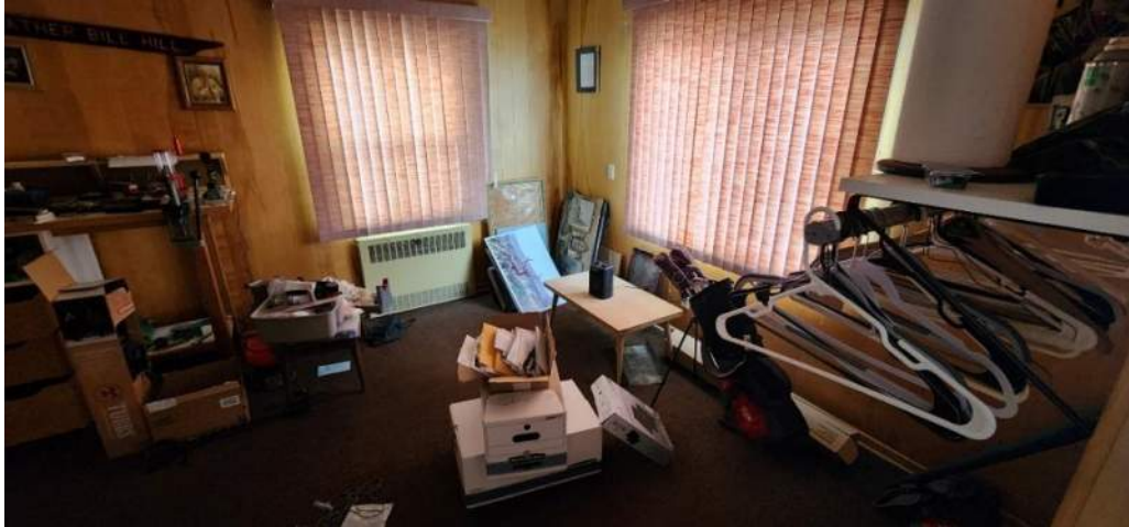
The offices within the Rectory have an older low-pile carpet. It does not appear to show significant failure, but does show wear in various areas.
