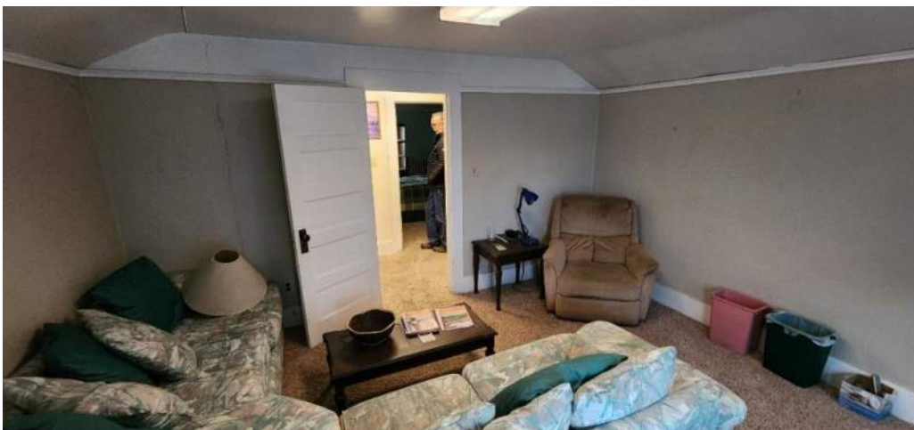
Lighting throughout is aged and should be upgraded throughout. Some signs of settling were visible in few walls of the upper level. Cracking does not show signs of continued growth and could be repaired.
