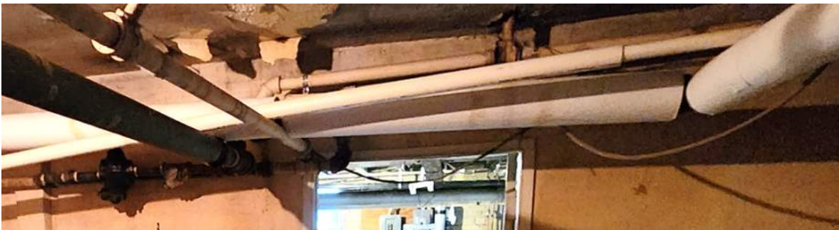
Significant staining on walls, peeling on ceiling, and other damages
