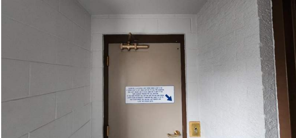
The door is equipped with a closer, latch, and handle. Without clear area adjacent to the door, a person in a wheelchair cannot operate the machine solo, it requires assistance.
