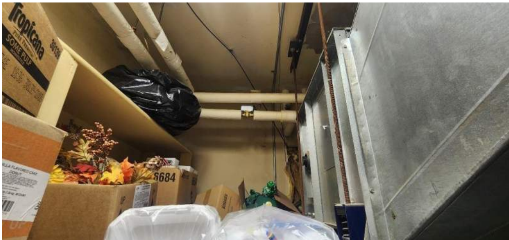
Storage within mechanical spaces is creating both hazard and serviceability issues for equipment.
