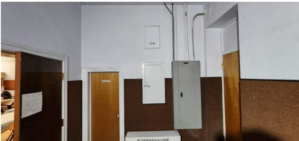
An upgraded electrical panel can be seen above a heater.
