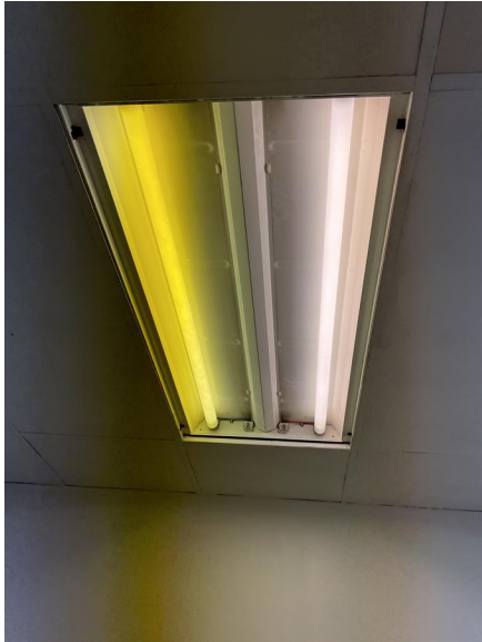
Fluorescent fixture missing lens
