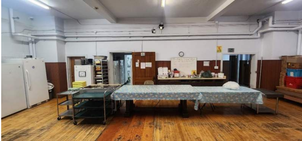
The floor is worn and requires repair for sanitary use within an eating establishment.
