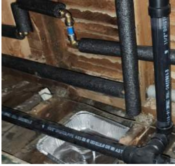
Plumbing w/ drip pans
