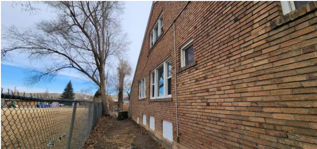
Repointing of the brick is necessary on the original Rectory. Where some bricks are excessively worn or damaged, replacement of similar type should be considered.
