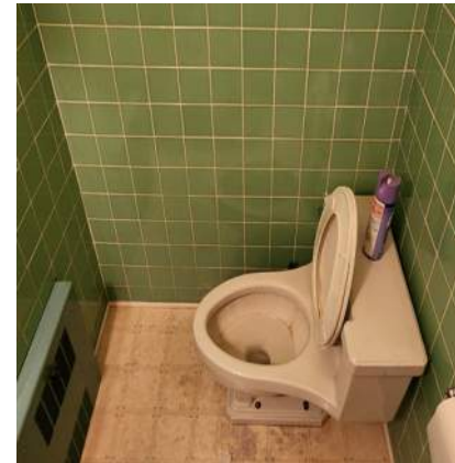
Undersized bathroom at offices
