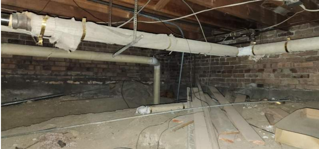
The basement turns to a crawlspace at the southern end of the original Rectory structure. Sections of insulation wrap are damaged on pipes, or missing at some locations.
