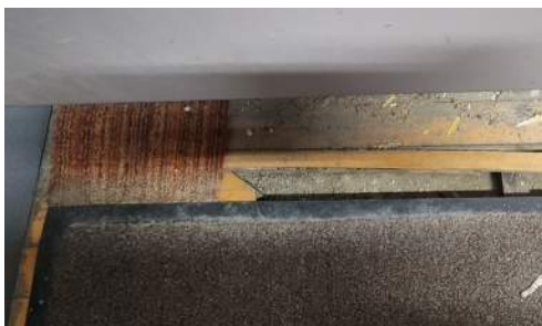
Exposed dirt under removed plank
