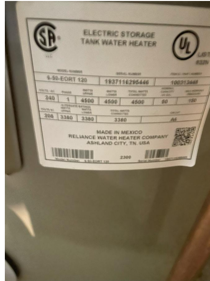
Rectory - 50 gallon Electric Water Heater
