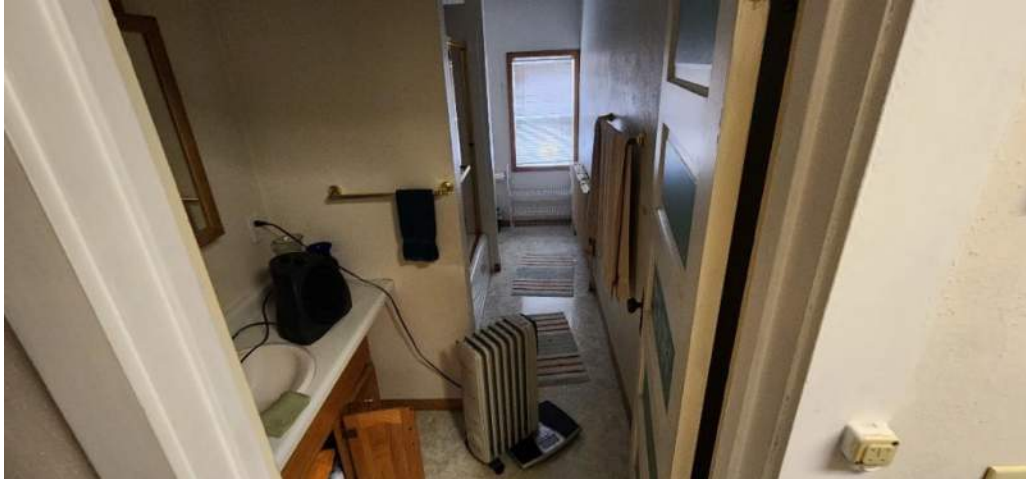
Bathroom is in decent overall condition. There are devices that have been abandoned and should be removed in their entirety. There is some cracking visible on walls.
