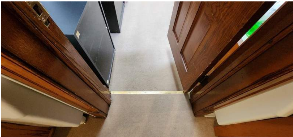
A step in the doorway is present from Altar to Sacristy without proper landing on swing side.
