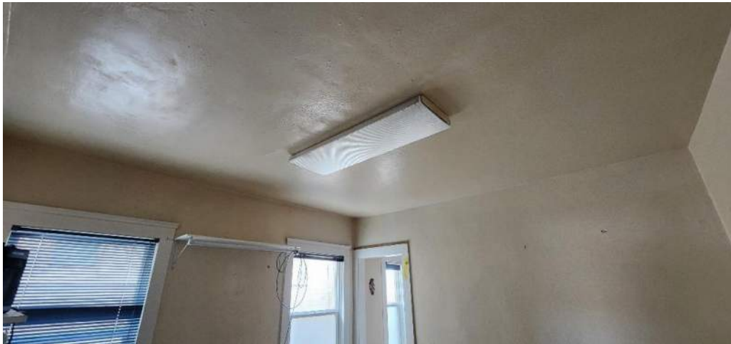
Lighting is aged and should be replaced/upgraded.
