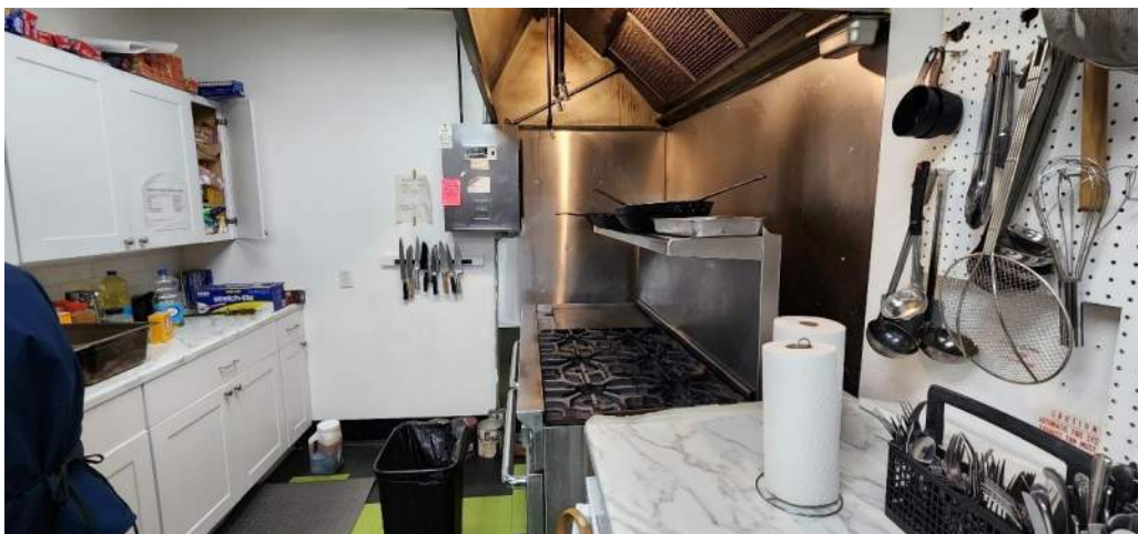
The grease hood has required fire suppression built in.
