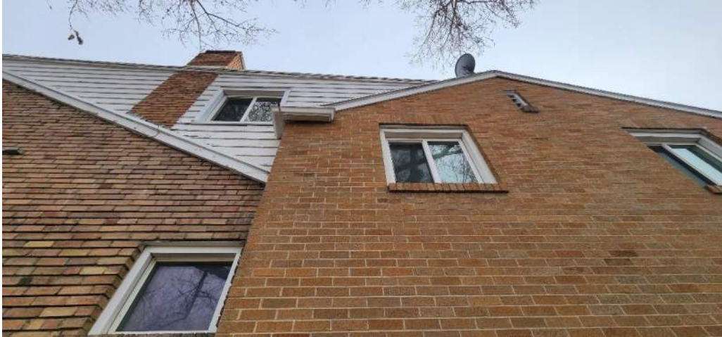
The view of the infill construction above. This also creates a conduit for moisture runoff where all three systems tie together, accelerating the wear on the brick and materials below.
