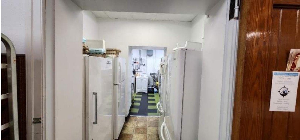
Access to the kitchen obstructed by a number of fridges/freezers for cold storage. The flooring is torn and create sanitary concerns for spills, etc. Flooring should be non-slip, non-porous, and resistant to grease and other chemicals/fluids.
